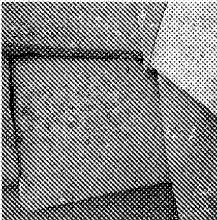
Example of small dropping found on a roof tile beside hanging tiles
