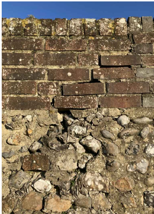
Photo 2 - existing cracking and damage to the wall in the area proposed to be removed and reconstructed
