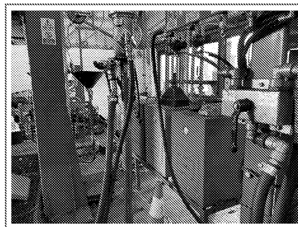
Waste fluid extraction system within the depollution building
