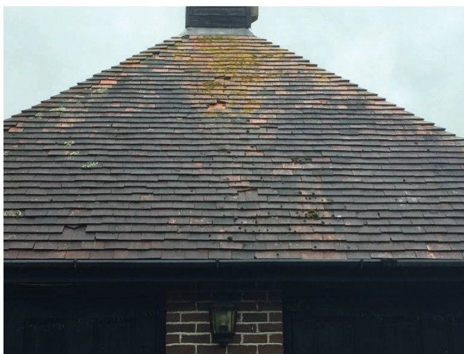
Photograph 5 Gaps under roof tile on eastern elevation of Building 2
