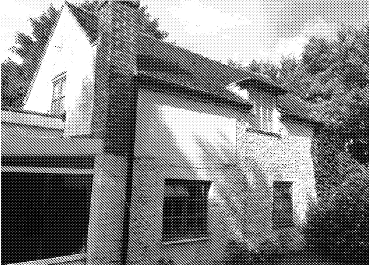
Figure 20. The south and eastern faces of Nightingale Cottage which has a hand-made clay tiles gable roof with numerous gaps.
