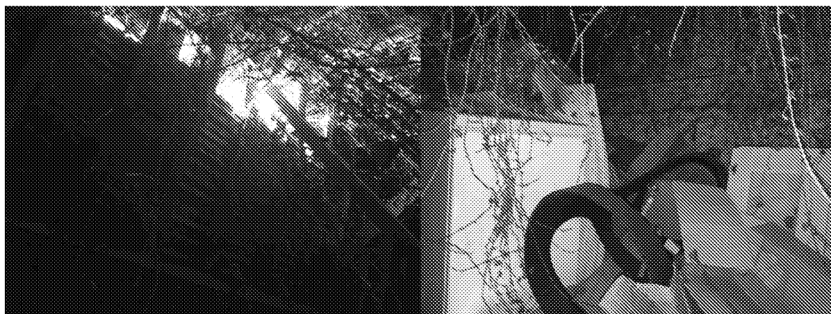
Figure 25. Internal aspect of the small barn used for storage with cobwebbing and ivy growth and numerous gaps between the roof tiles.
