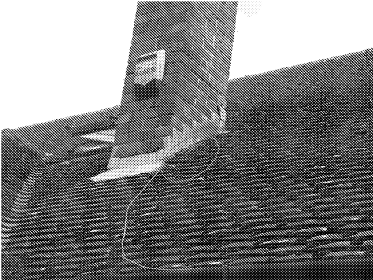
Figure 16. A small number of lifted roof tiles around the chimney on the southern face
