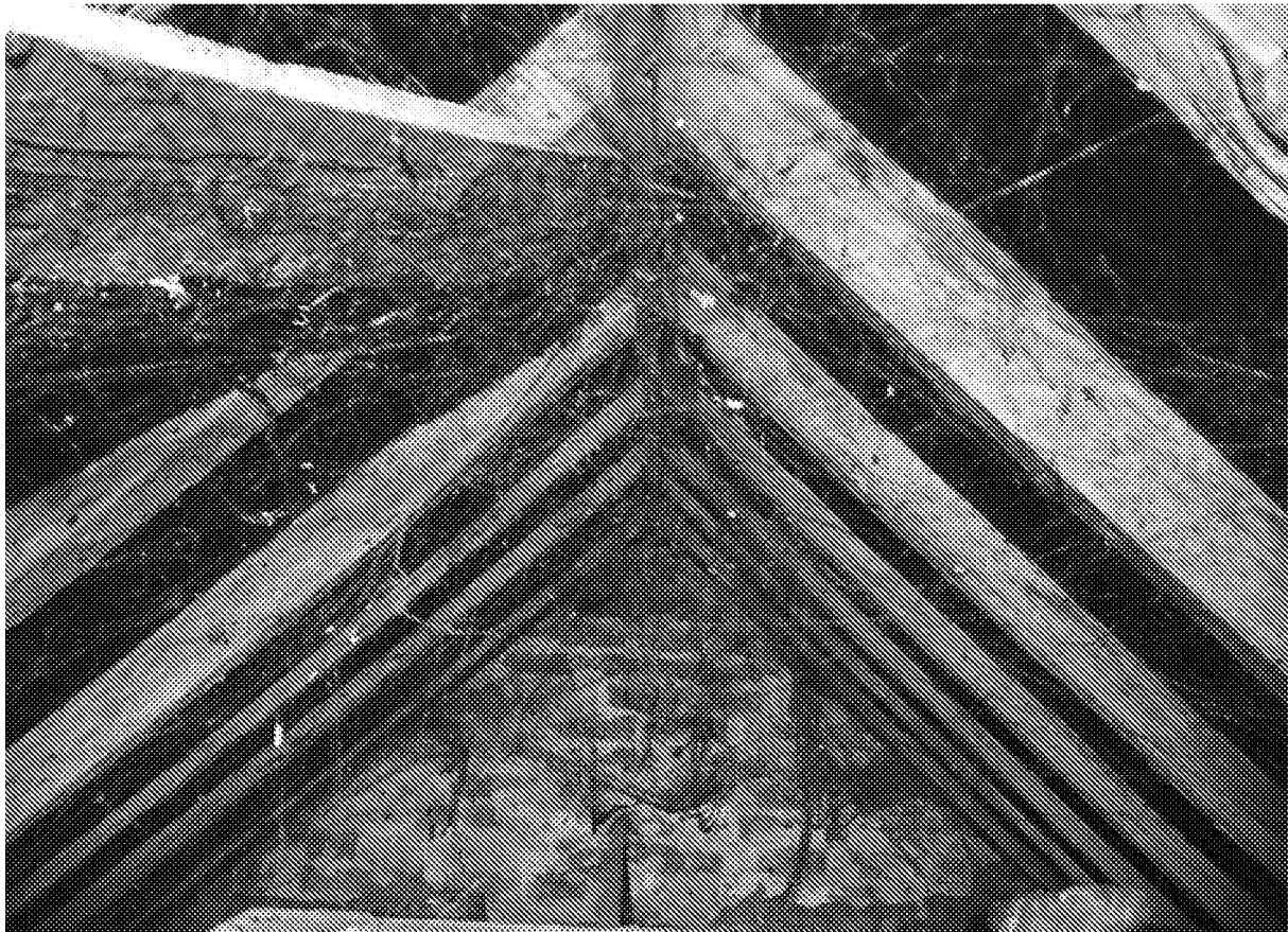
Figure 23. The void within Nightingale Cottage which is very heavily cobwebbed.
