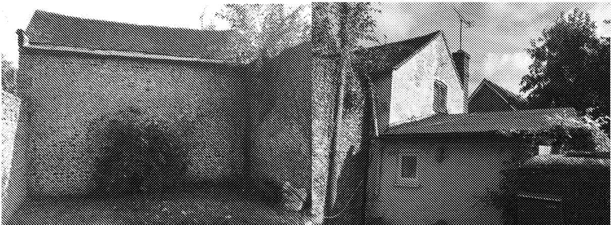
Figure 21. Western faces of Nightingale Cottage with a bitumen lined section.
