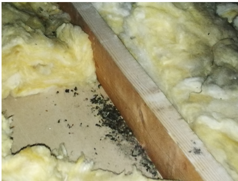
Figure 7. Collection of old bat droppings within the loft space of the bungalow.
