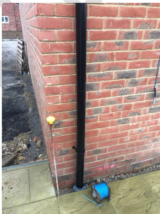
Rainwater pipe at Plot 8
