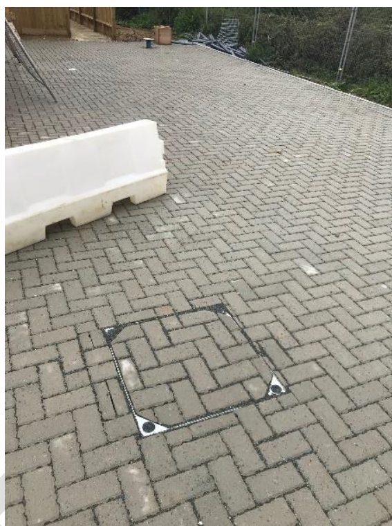
Recessed cover for the catchpit at Plot 20 and Plot 21 shared driveway
