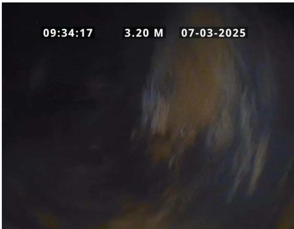
Finish node, manhole, reference: PS169
