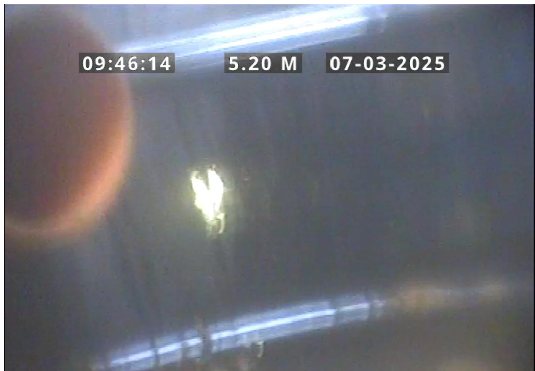
Finish node, manhole, reference: PS169
