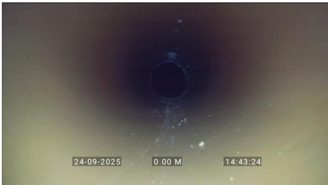
Start node, manhole, reference: PSCP67
