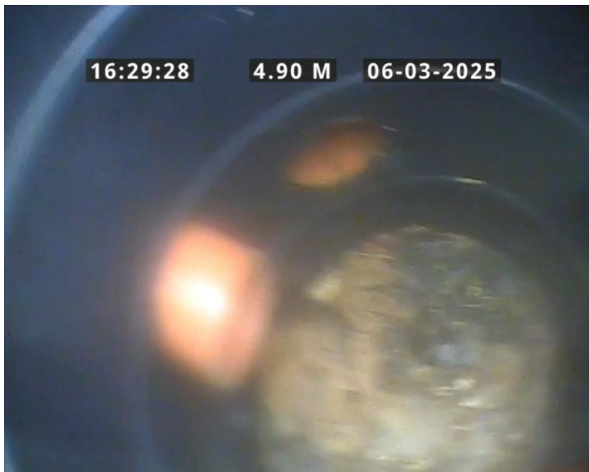
Finish node, manhole, reference: PSCP038
