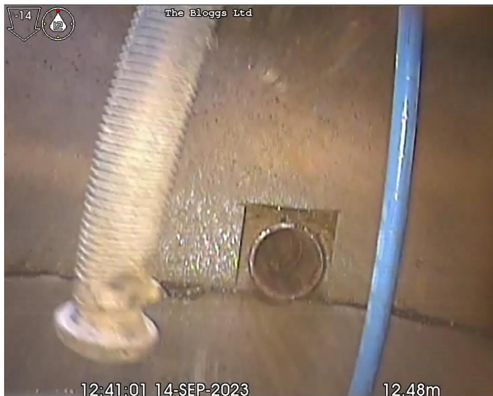
Finish node, manhole, reference: S6
