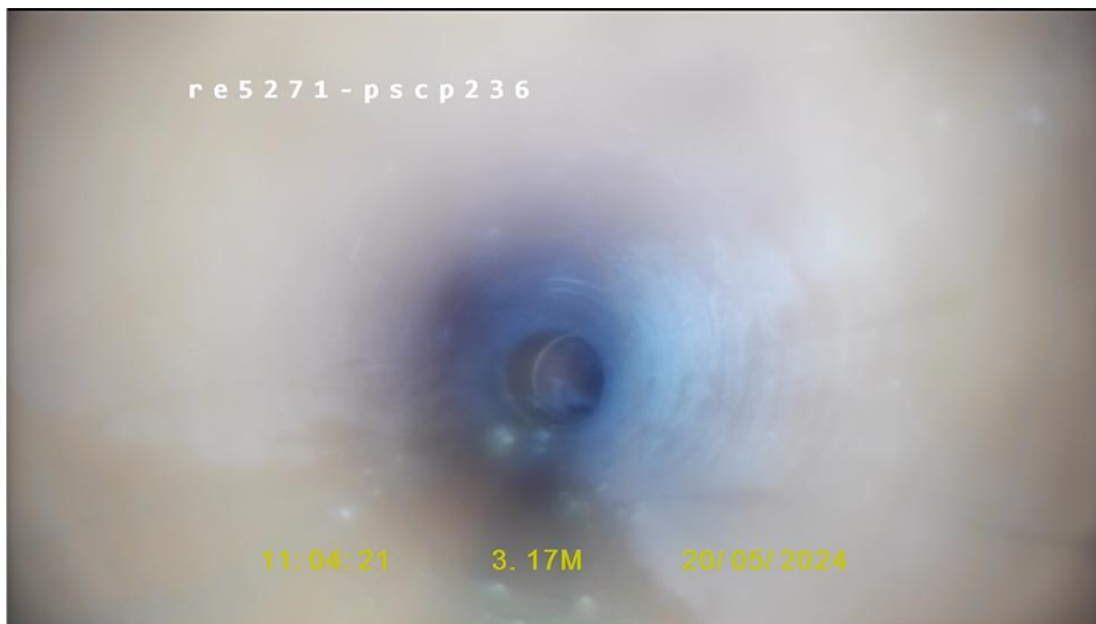
Finish node, manhole, reference: PS235
