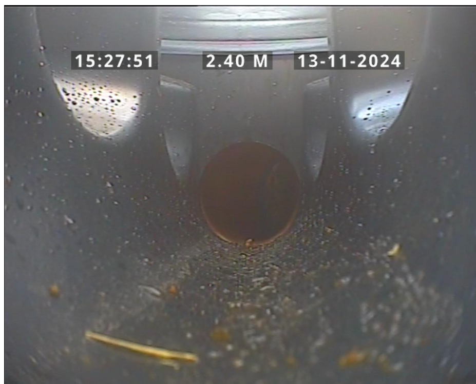
Finish node, manhole, reference: PS254
