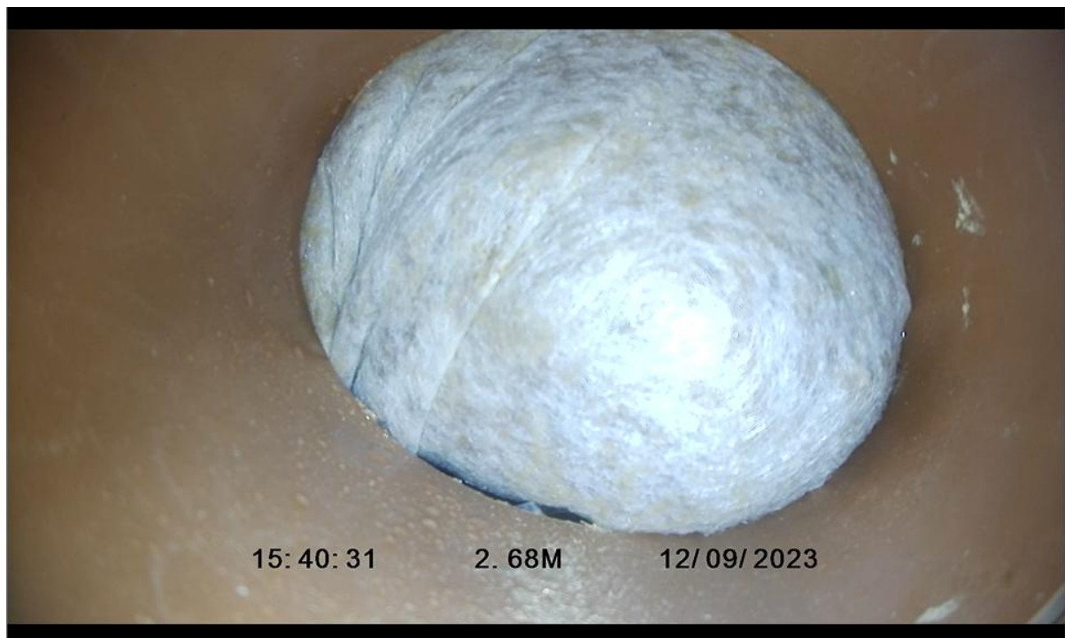
Finish node, manhole, reference: SA48
