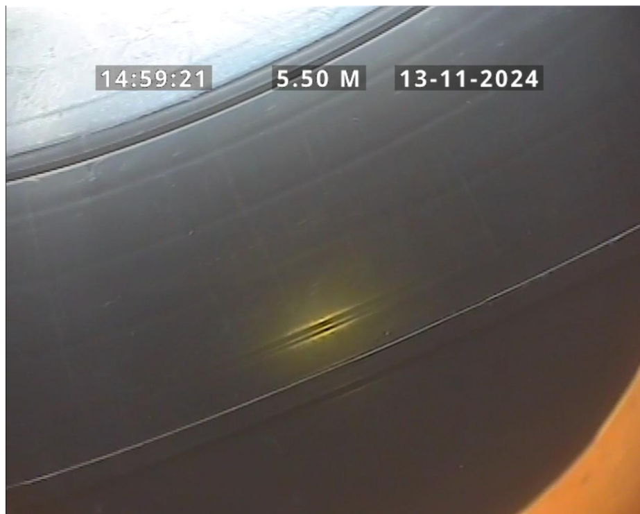
Finish node, manhole, reference: PSCP236
