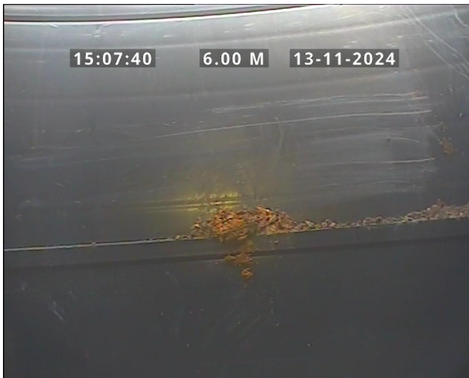
Finish node, manhole, reference: PSCP240
