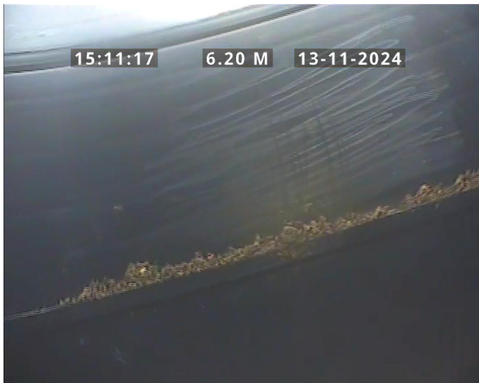
Finish node, manhole, reference: PSCP335
