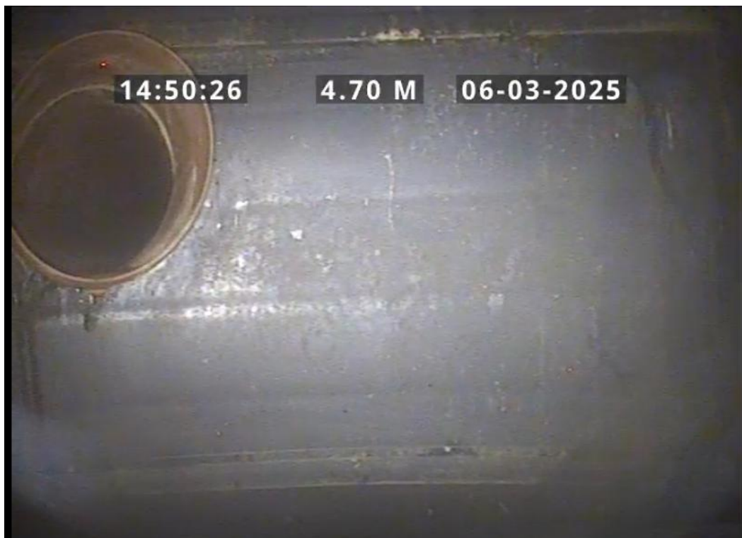
Finish node, manhole, reference: PS342
