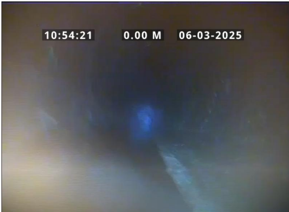
Start node, manhole, reference: PS209
