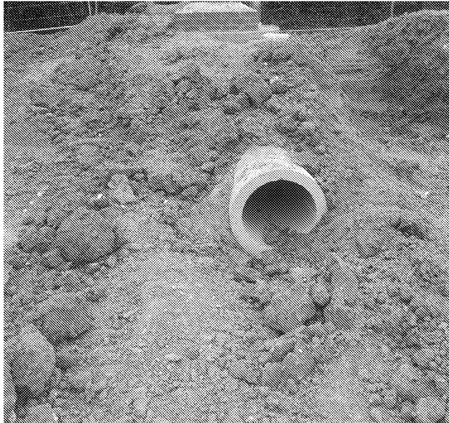
Manhole And Its Connector Pipe
