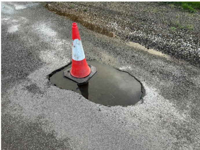
Plate 19 Flooding in Church Road – 28 th March 2026 – resultant highway damage
