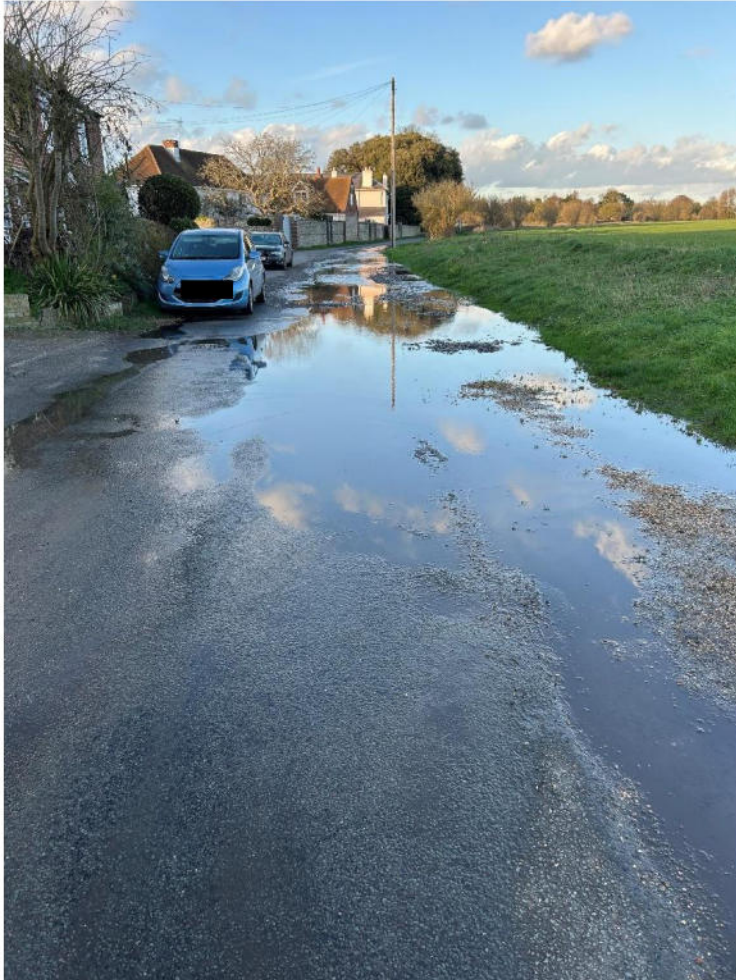
Plate 18 Flooding in Church Road – 28 th February 2026
