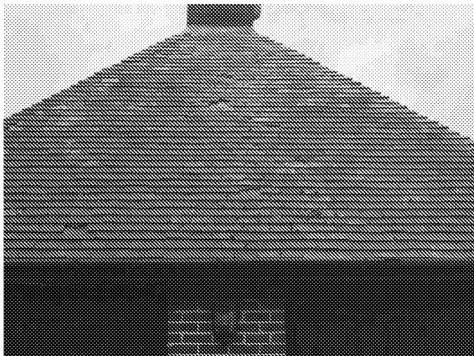
Photograph 5 Gaps under roof tile on eastern elevation of Building 2
