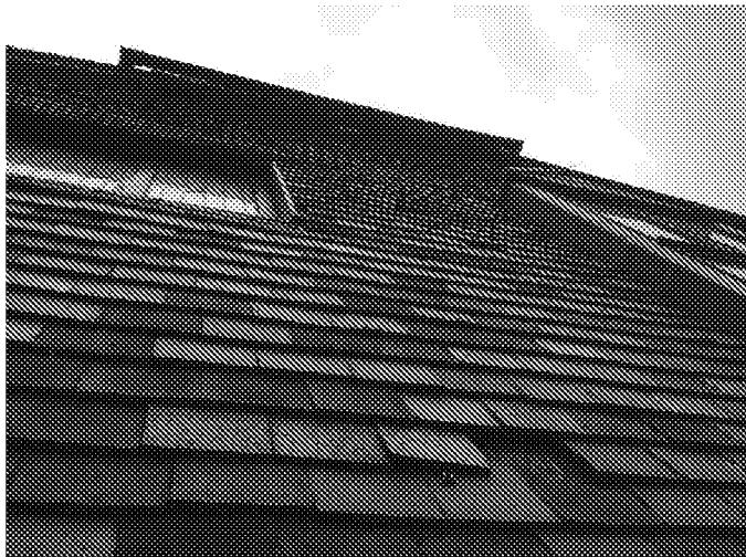
Photograph 6 Gaps under hanging tiles on eastern elevation of Building 2
