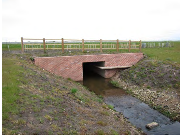
Figure 2- Culvert with Ledges for Mammal Passage
