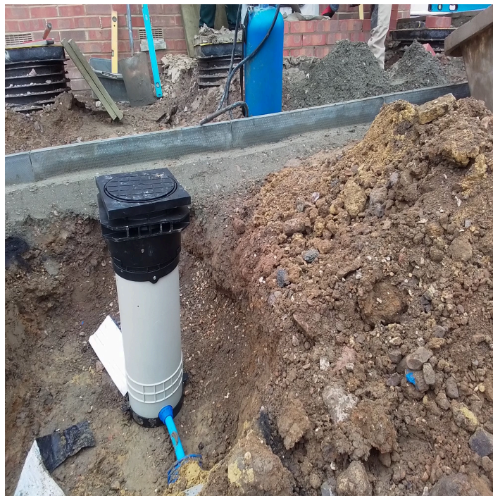
Photo of Water Meter box / Boundary Box
