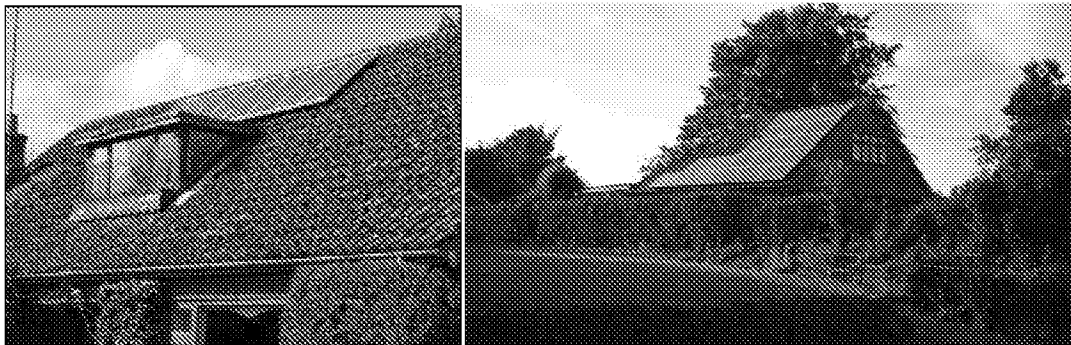
Figure 4: Standard PV panels installed on a houses in Berkshire and Oxfordshire
