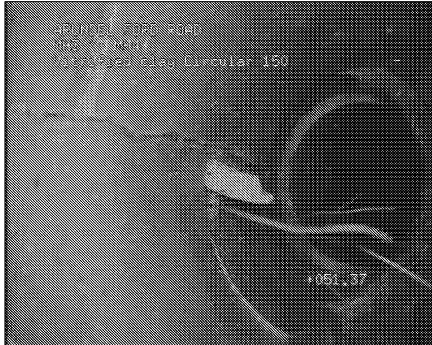
Photo: 3_3_108_A.JPG 51.37m, Fracture, multiple, from 6 to 6 o'clock
