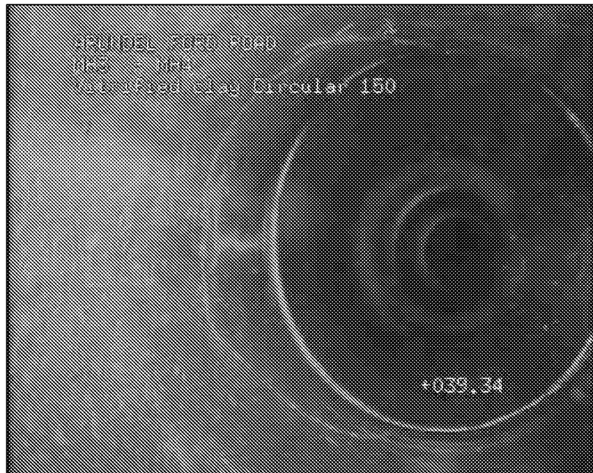
Photo: 3_3_85_A.JPG 39.34m, Fracture, multiple at joint, from 7 to 5 o'clock
