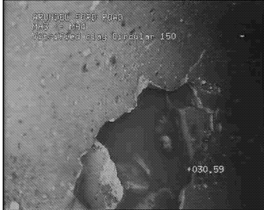
Photo: 3_3_72_A.JPG 30.59m, Hole in drain/sewer, at 6 o'clock
