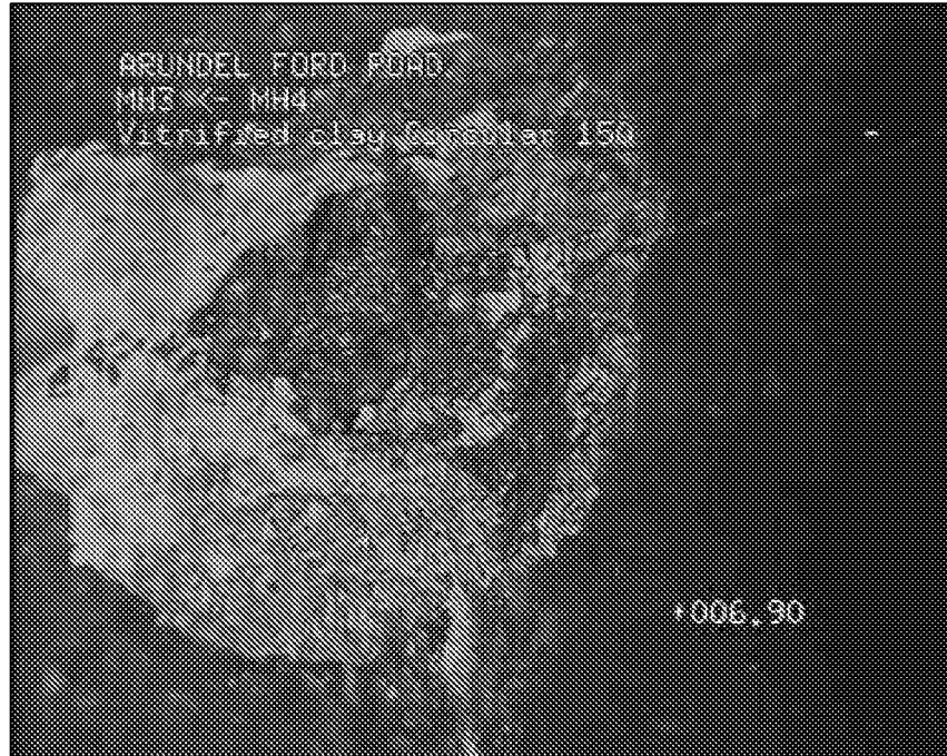
Photo: 3_3_40_A.JPG 6.9m, Hole in drain/ sewer, at 12 o'clock
