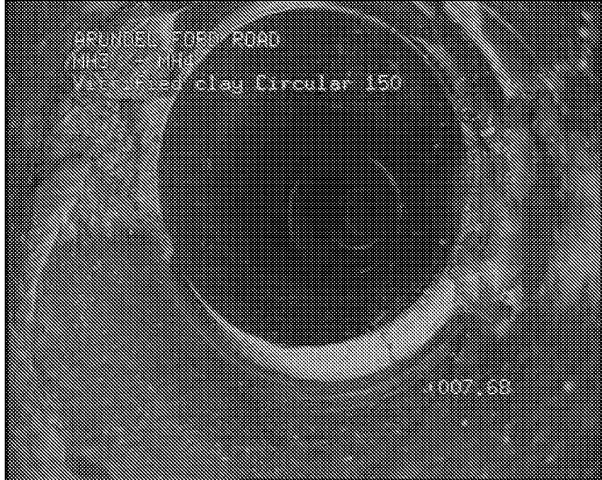
Photo: 3_3_43_A.JPG 7.68m, Fracture, multiple at joint, from 6 to 6 o'clock
