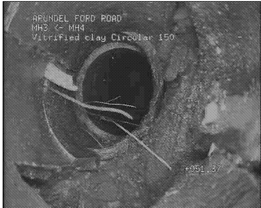
Photo: 3_3_107_A.JPG 51.37m, Hole in drain/sewer, from 3 to 9 o'clock
