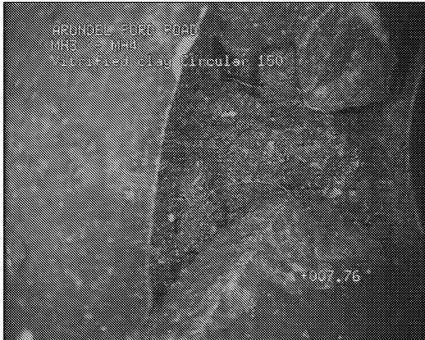
Photo: 3_3_44_A.JPG 7.76m, Hole in drain/sewer at joint, at 12 o'clock
