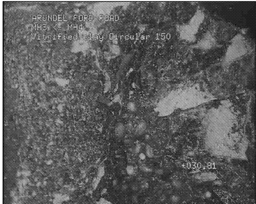
Photo: 3_3_73_A.JPG 30.81m, Hole in drain/sewer, at 12 o'clock
