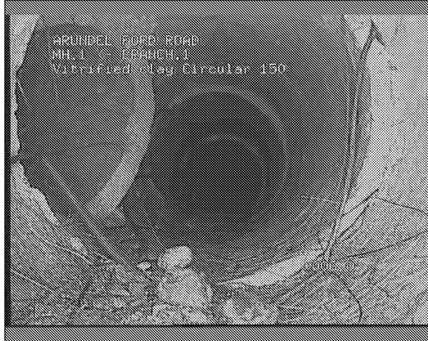
Photo: 4_4_18_A.JPG 6m, Connection intruding, at 9 o'clock, diameter 100mm, intrusion 25%
