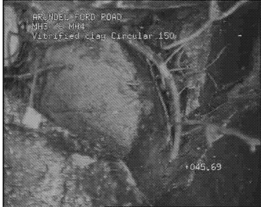
Photo: 3_3_94_A.JPG 45.69m, Hole in drain/sewer, from 11 to 12 o'clock
