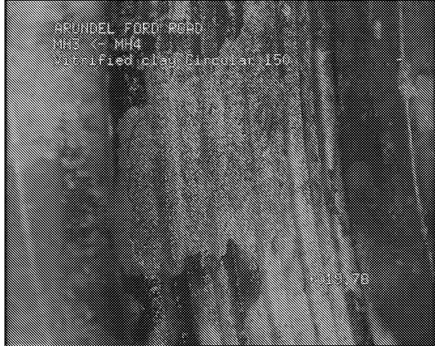
Photo: 3_3_60_A.JPG 19.76m, Open joint, medium
