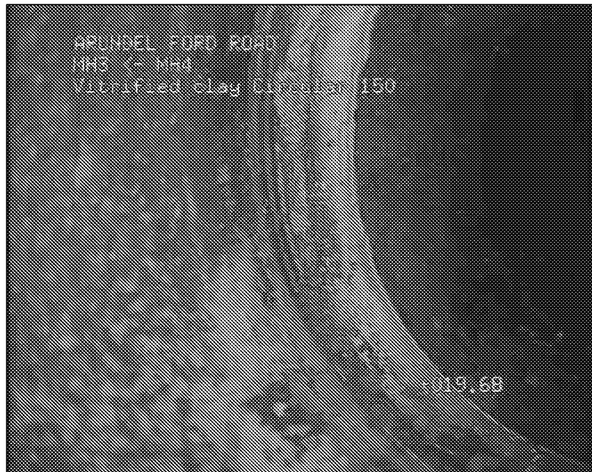
Photo: 3_3_59_A.JPG 19.67m, Joint displaced, medium
