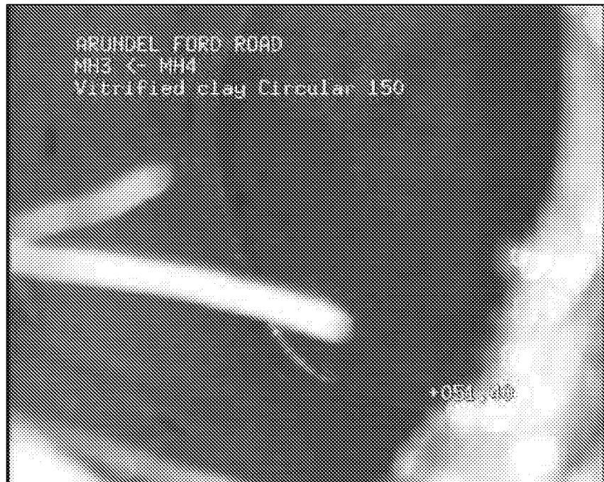
Photo: 3_3_113_A.JPG 51.4m, General remark
