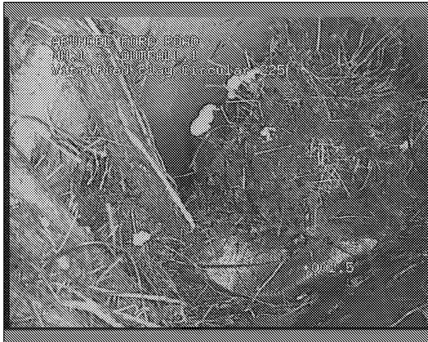
Photo: 6_6_54_A.JPG 1.5m, Roots, tap at joint
