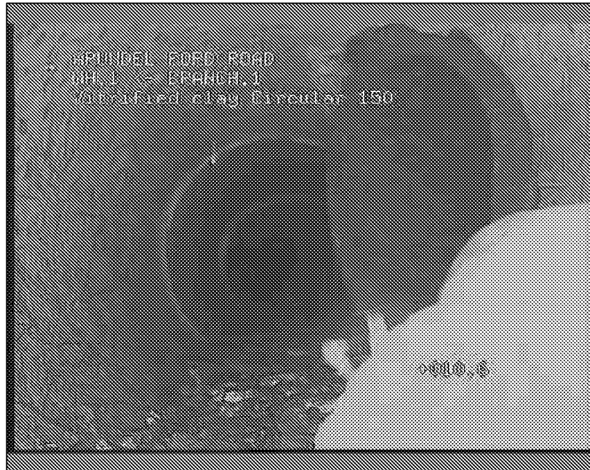
Photo: 4_4_21_A.JPG 10.6m, Connection intruding, at 3 o'clock, diameter 150mm, intrusion 30%
