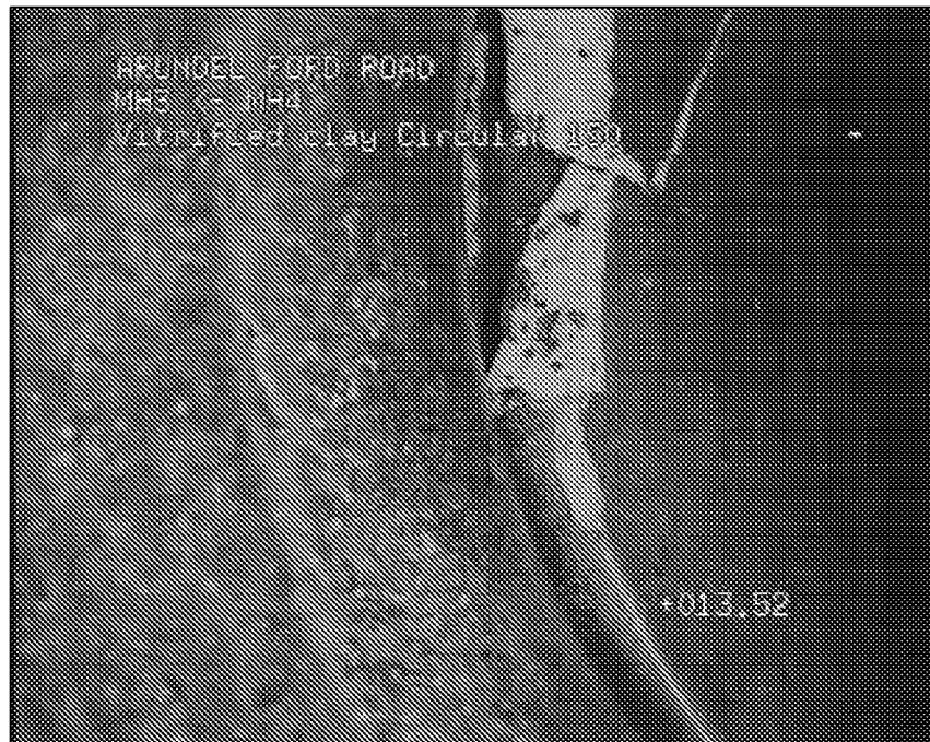
Photo: 3_3_49_A.JPG 13.52m, Hole in drain/sewer at joint, from 11 to 12 o'clock
