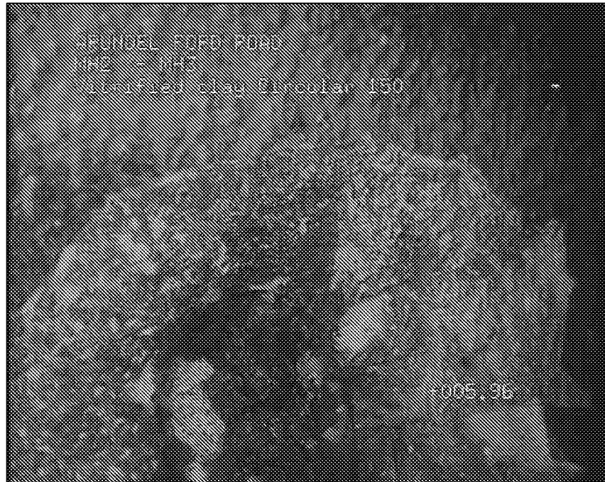
Photo: 1_1_19_A.JPG 5.95m, Hole in drain/ sewer, at 9 o'clock
