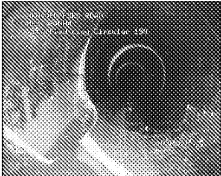
Photo: 3_3_27_A.JPG 0.6m, Broken pipe, from 5 to 7 o'clock
