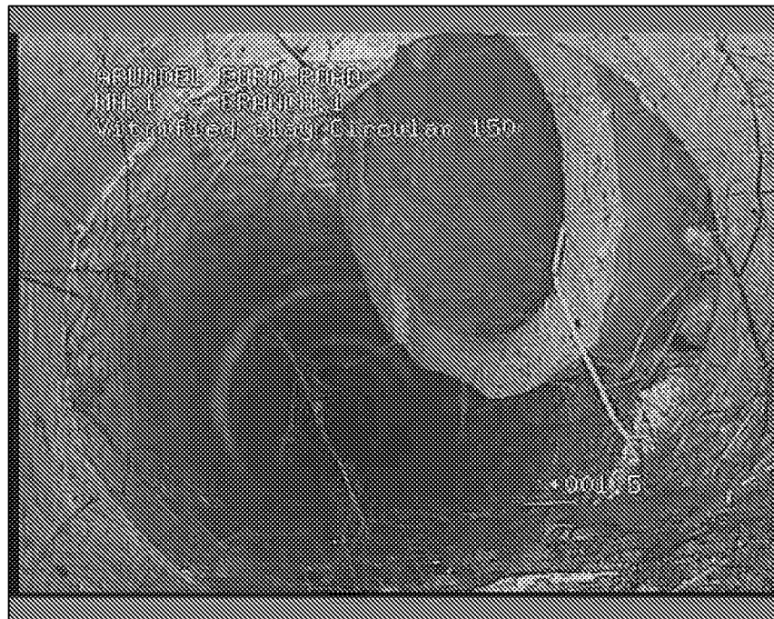
Photo: 4_4_17_A.JPG 1.5m, Connection intruding, at 2 o'clock, diameter 100mm, intrusion 40%
