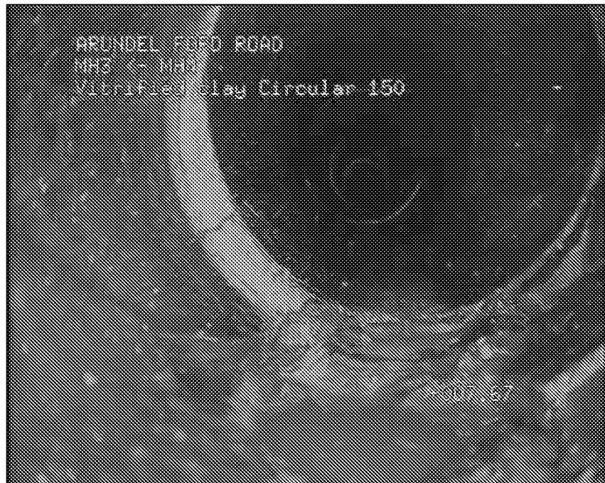
Photo: 3_3_42_A.JPG 7.67m, Hole in drain/ sewer at joint, at 6 o'clock
