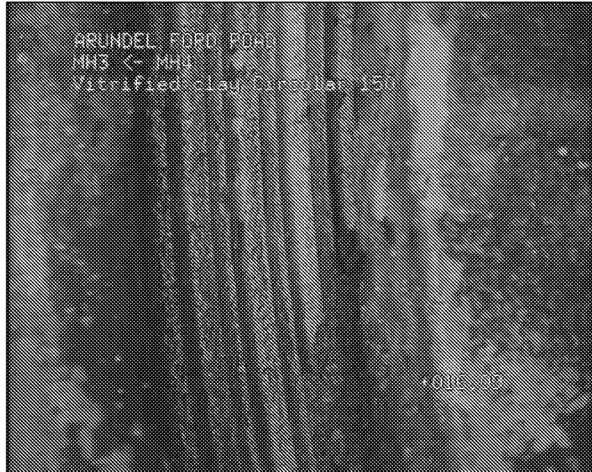
Photo: 3_3_57_A.JPG 16.09m, Open joint, medium
