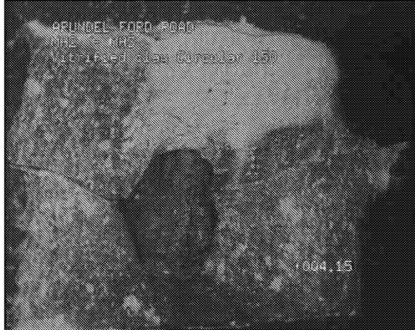
Photo: 1_1_14_A.JPG 4.15m, Hole in drain/ sewer, at 12 o'clock
