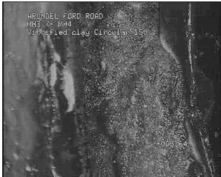
Photo: 3_3_35_A.JPG 3.64m, Open joint, medium
