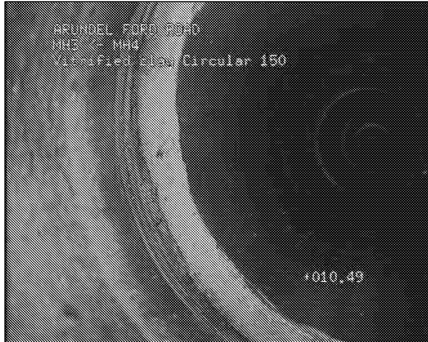
Photo: 3_3_46_A.JPG 10.49m, Joint displaced, medium
