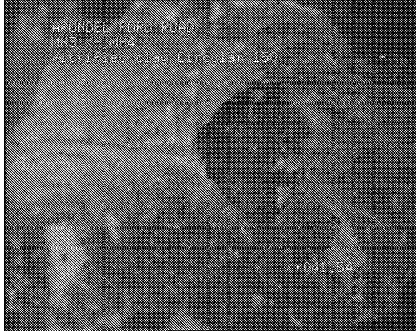
Photo: 3_3_90_A.JPG 41.54m, Hole in drain/sewer, from 11 to 12 o'clock
