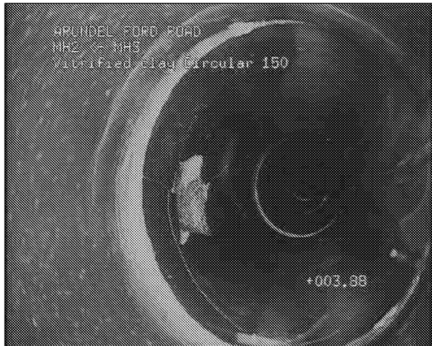
Photo: 1_1_13_A.JPG 3.86m, Fracture, multiple at joint, from 7 to 5 o'clock
