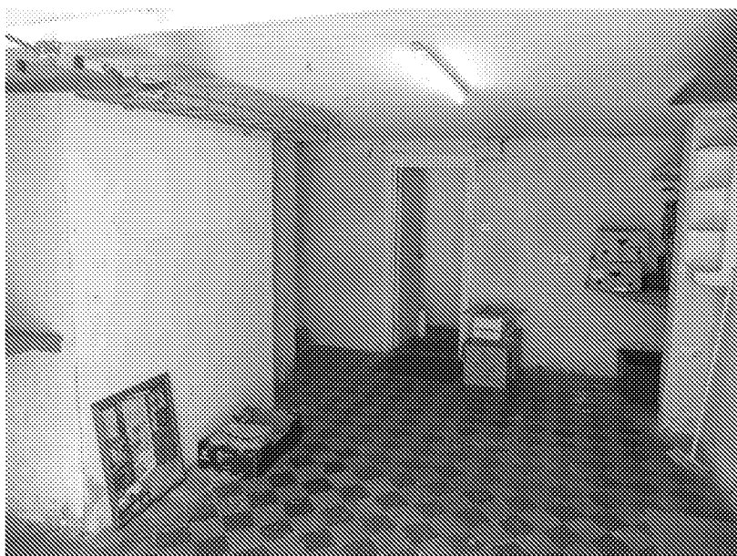
Photo 8 – Garage area within basement, with limited headroom.
