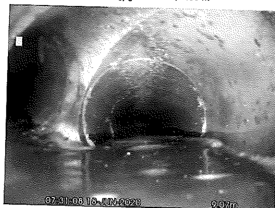
INLET X_22688d2d-cd74-47d9-8b74-29ab69b13bb5_20200623_224 711_563.jpg, 00:01:12, 9.07 m
