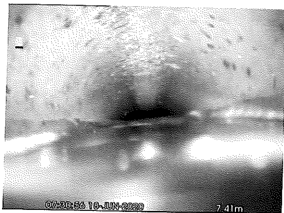
INLET X_7aaaa846-527c-4dfb-9265-dfd9de3c1ecc_20200623_2246 38_719.jpg, 00:01:00, 7.41 m
