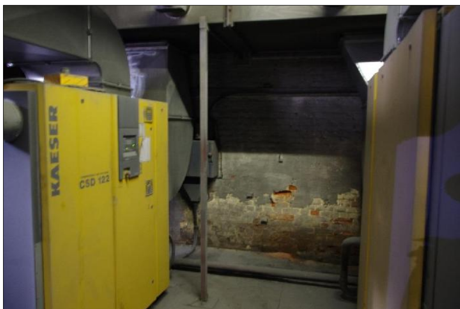
Plate 12: Plant room in south room contains modern industrial blast cleaning processes.
