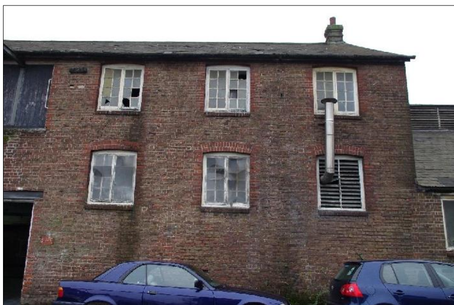
Plate 4: View looking west towards northern extent of two-storey range where casement 16-light segmental arch timber-framed windows have been damaged, or replaced with modern modern louvers and plant.
