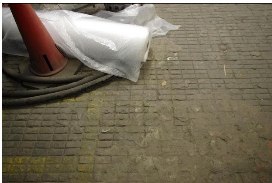
Plate 10: Engineering brick floor patched up with modern concrete.
