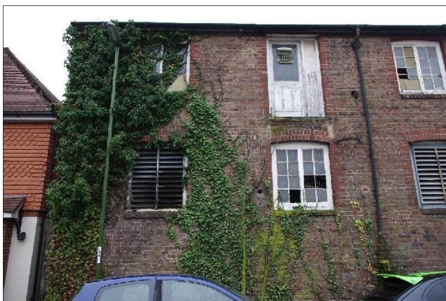
Plate 2: View looking west towards southern extent of two-storey range. The first-floor single-leaf door has had its original stair access removed. Vegetation is prevalent on this part of the building and damaged downpipes have resulted in rising damp.
