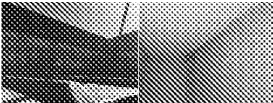
Image – Photos - Arundel Town Hall – Cement Render and internal damp
