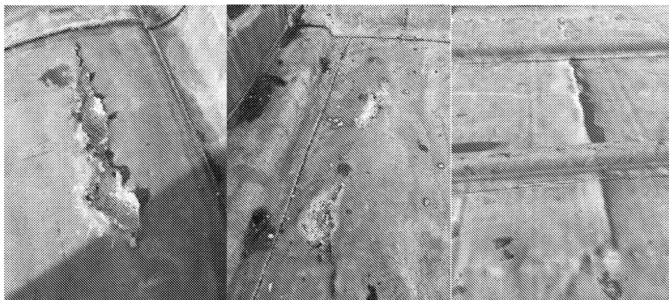
Splits in lead sheet
