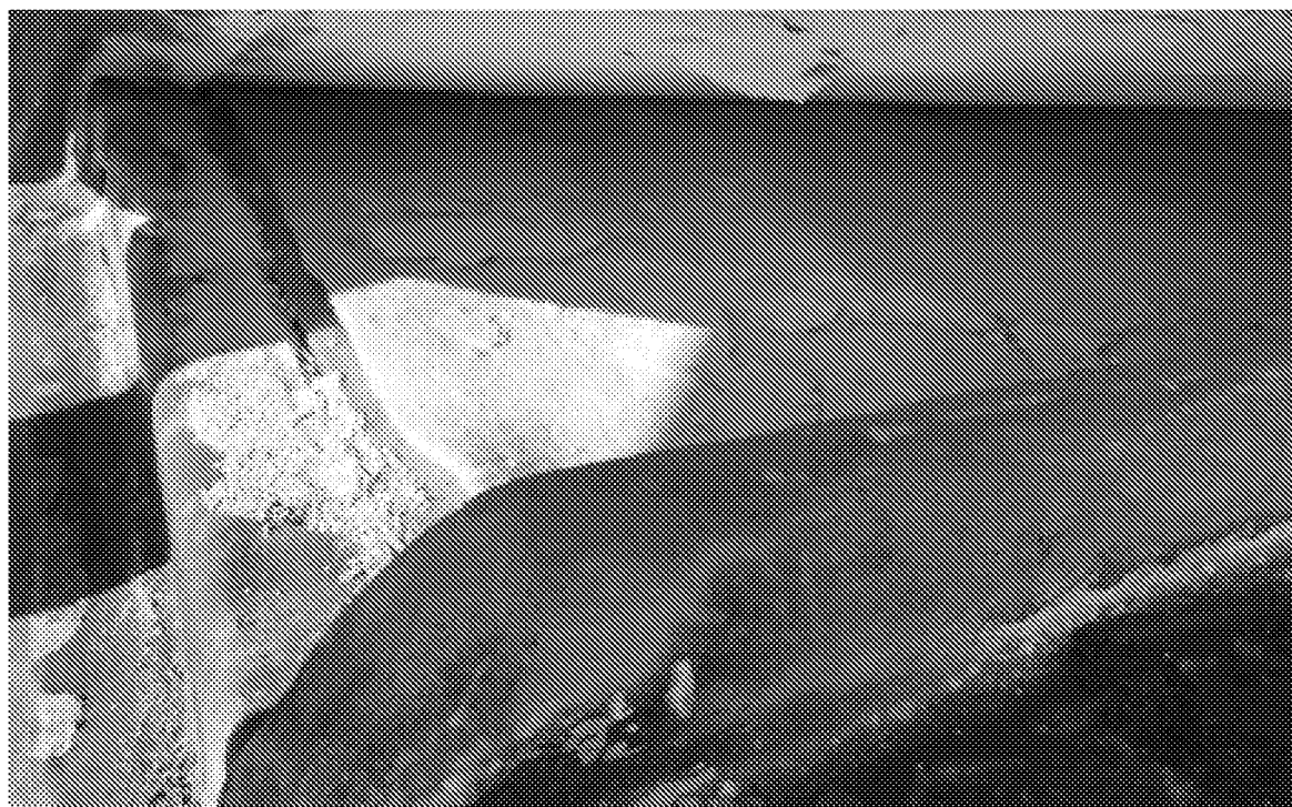
Image – Photo - Arundel Town Hall – Underside Lead Corrosion & geotextile underlay
