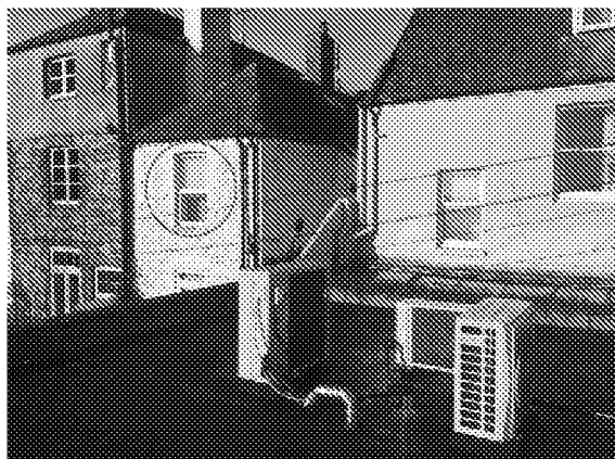
Figure 7: NSR and Plant (cooler not yet moved)
