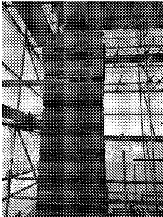
Photograph 2: Packer in chimney joint
