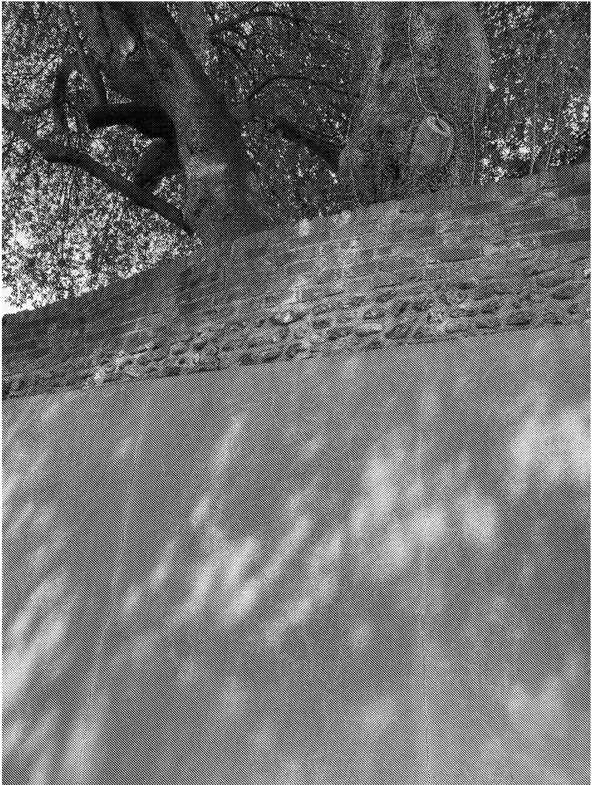
Figure. 6 Illustrating multipule cracks in the wall.
