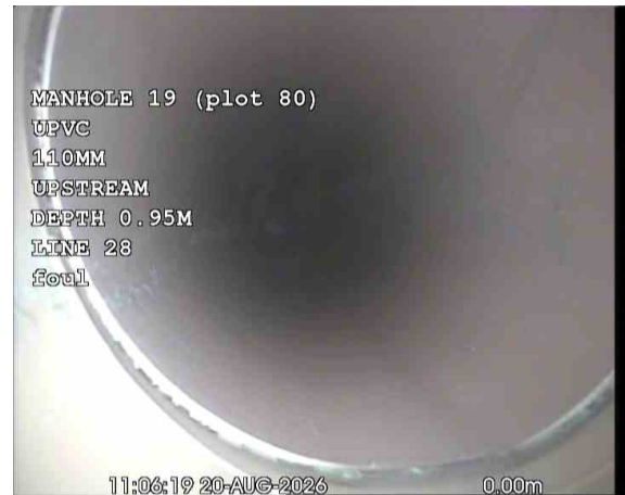
W_CX_e79d9ecf-1e93-4095-96e0-de79c73465f6_20260917_173242_989.jpg, 00:00:14, 0.00 m Water level, 0% of the vertical dimension
