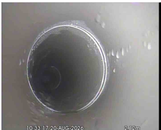
KIT. SINKX_4c4615d5-8afe-46fe-abfa-9437e60ddb6a_20260917_172106_901.jpg, 00:01:12, 2.12 m Line deviates left
