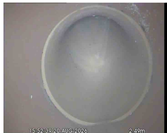
BASINX_af4bf942-a14d-4ed3-81e3-fa4dacbd8225_20260918_093726_384.jpg, 00:00:30, 2.49 m Line deviates up, REST BEND
