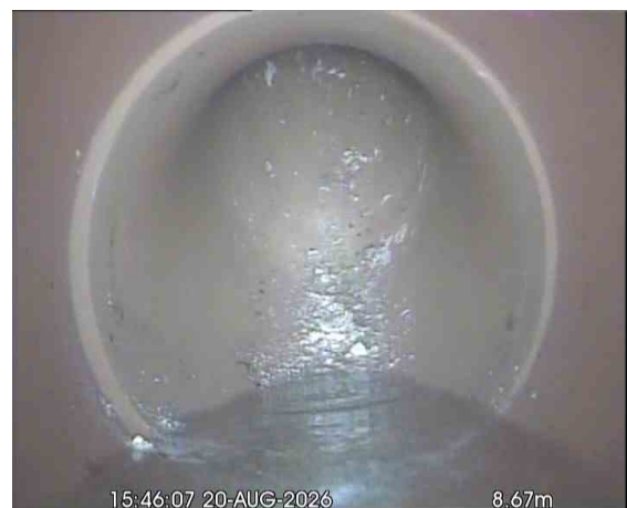
UTIL. SINKX_b7ee2398-778b-4f67-8334-e8b9281de2ef_20260918_093422_014.jpg, 00:01:37, 8.67 m Line deviates up, REST BEND
