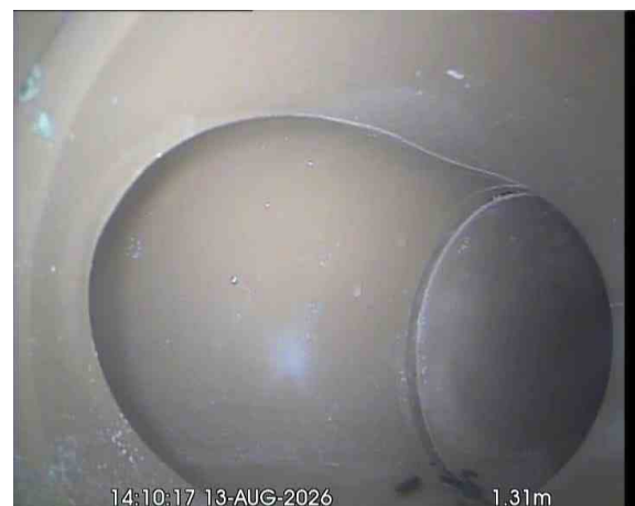
MH16X_428f2b95-b001-412b-abc9-27e4679198db_20260917_170720_699.jpg, 00:00:41, 1.31 m Finish node, major connection without manhole, reference: BLIND JUNCTION - JOINS SECTION 22 (S22)
