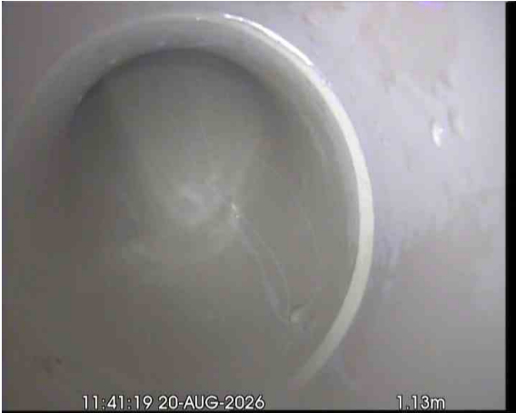
SVPX_e427ca2a-107a-4ea9-a0da-e44bbd509246_20260917_175526_581.jpg, 00:01:08, 1.13 m Line deviates up, REST BEND
