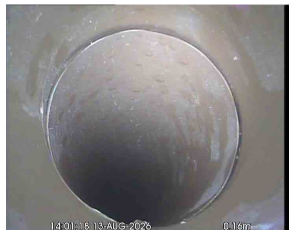
MH15X_44809b83-cdf5-49f5-81d1-d98588b7e15e_20260917_170146_168.jpg, 00:00:31, 0.16 m Line deviates down
