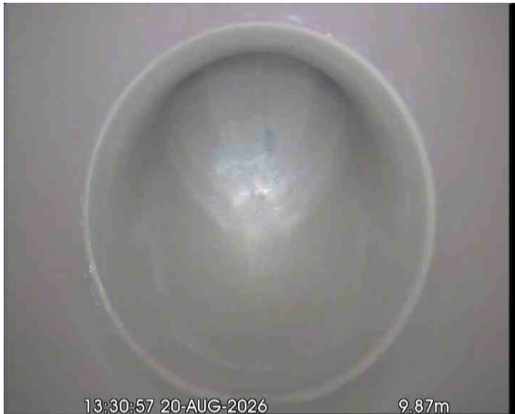
SVPX_756a6aed-3973-4003-ae3d-e4813c50bb8d_20260917_184639_991.jpg, 00:01:10, 9.87 m Line deviates up, REST BEND
