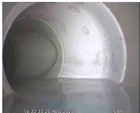
MH31X_115ecd48-0f7e-4833-8da0-a25af0dfec4b_20260918_094749_553.jpg, 00:00:38, 1.68 m Line deviates left
