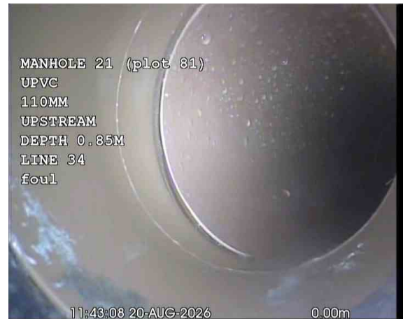
BASINX_2e006caf-2029-45e4-9114-5515bd78bad2_20260917_175739_095.jpg, 00:00:22, 0.00 m Water level, 0% of the vertical dimension
