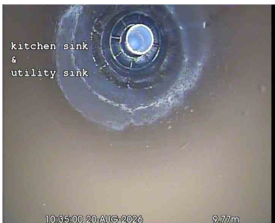
KIT. SINKX_922ef9a8-3312-49c9-a29f-98dec6e21b2e_20260917_172141_099.jpg, 00:02:14, 9.77 m Finish node, major connection without manhole, reference: KITCHEN & UTILITY SINK
