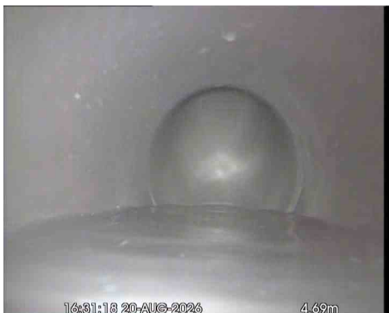
SVPX_c6ebe67c-cb53-4259-b9f6-362d6ffde17f_20260918_094512_423.jpg, 00:01:22, 4.69 m Water level, 15% of the vertical dimension
