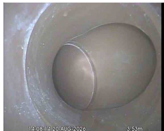
MH27X_e1fb74e4-a880-4f38-96f8-fdb0901240fd_20260917_190405_482.jpg, 00:00:58, 3.53 m Finish node, major connection without manhole, reference: BLIND JUNCTION - JOINS SECTION 50 (S50)
