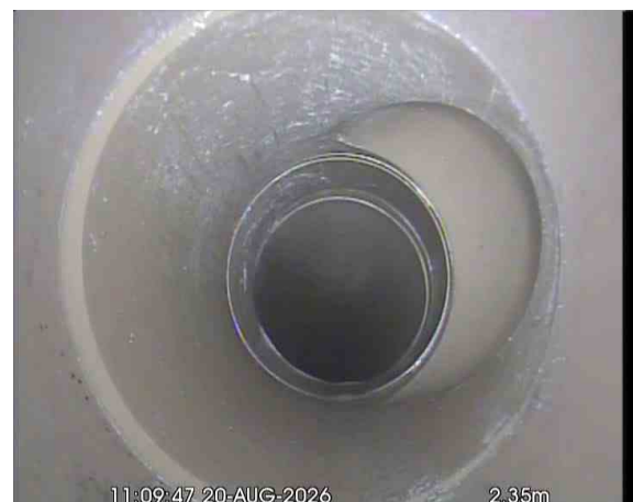
MH19X_51f7dcac-fc35-4f2e-b122-b16cd6f3f567_20260917_173523_814.jpg, 00:00:48, 2.35 m Junction at 3 o'clock, diameter: 110mm, SECTION 26 (S26)
