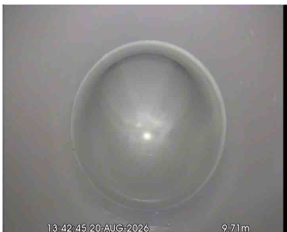
CAPPED OFFX_9f5d1a94-85fc-4e28-803a-5e62180bdc04_20260917_185346_439.jpg, 00:01:35, 9.71 m Line deviates up, REST BEND
