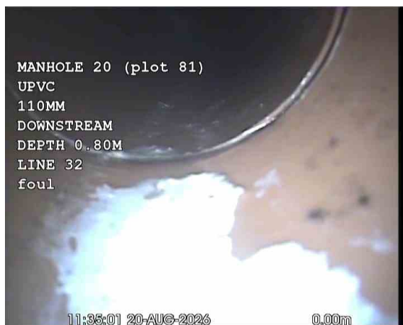
MH20X_addaded3-ee16-4463-8b45-4729e01231ef_20260917_175245_849.jpg, 00:00:30, 0.00 m General remark, **PLOT 81**
