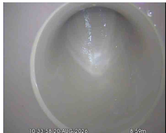
KIT. SINKX_ef349aab-60ba-42da-a7c8-8815dd824d1a_20260917_172122_502.jpg, 00:01:52, 8.59 m Line deviates up, REST BEND
