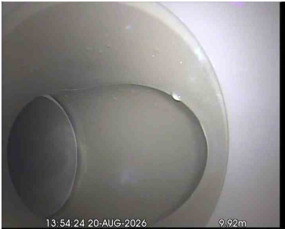
MH26X_3f77b62a-d4bf-4e03-9595-01586d9bcbe4_20260917_185934_254.jpg, 00:02:16, 9.92 m Finish node, major connection without manhole, reference: BLIND JUNCTION - JOINS SECTION 9 (S9)
