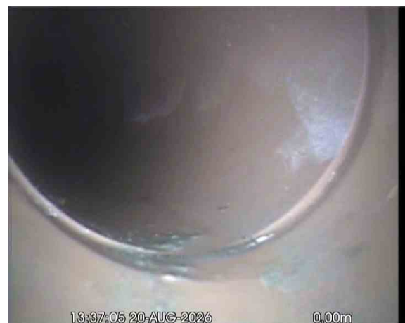
MH25X_bb028413-274f-412d-8ed7-1395f1435ce7_20260917_185029_539.jpg, 00:00:27, 0.04 m Line deviates left
