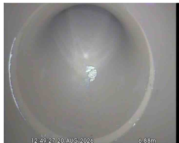
UTIL. SINKX_394e542c-b4db-432c-b100-f1df7faa1ed8_20260917_183603_212.jpg, 00:00:45, 6.88 m Line deviates up, REST BEND
