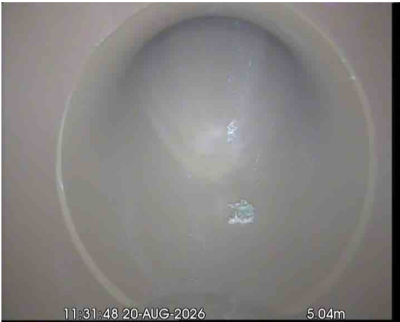
UTIL. SINKX_fb20255c-8285-4bca-80fd-bfd51da69a61_20260917_175107_919.jpg, 00:00:45, 5.04 m Line deviates up, REST BEND
