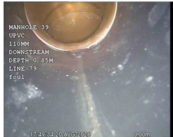
MH39X_b1249d83-7826-4e8b-8467-5343a7954b2a_20260918_103447_420.jpg, 00:00:23, 0.00 m Water level, 0% of the vertical dimension
