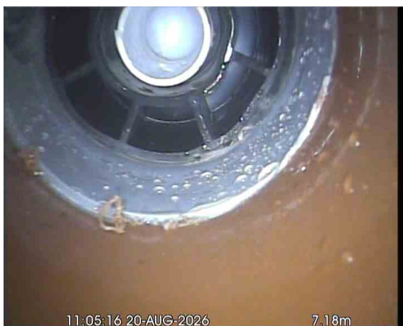
BASINX_de3d61d1-393a-4a94-8d68-8ebe88da30a0_20260917_173026_581.jpg, 00:01:22, 7.18 m Finish node, major connection without manhole, reference: BASIN
