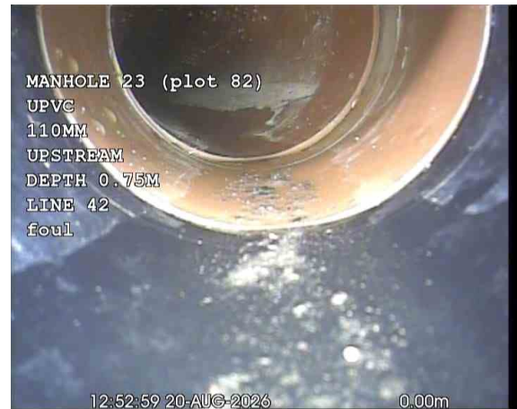
SVPX_ea48cf4c-2d03-450d-9455-21e902552caa_20260917_183717_262.jpg, 00:00:29, 0.00 m Water level, 0% of the vertical dimension
