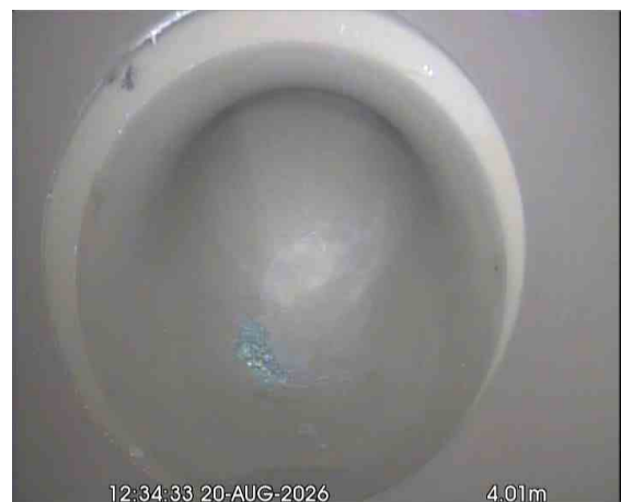
SVPX_12d30369-315d-4c96-89d5-d91a2ed2c29e_20260917_182841_615.jpg, 00:00:59, 4.01 m Line deviates up, REST BEND
