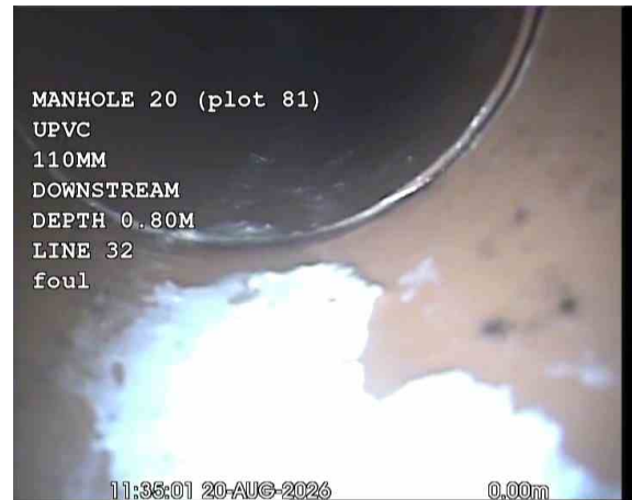
MH20X_096673fe-1158-46fa-b502-18065a805ed1_20260917_175235_014.jpg, 00:00:30, 0.00 m Water level, 0% of the vertical dimension
