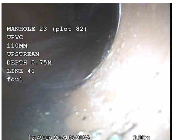
UTIL. SINKX_1c582c71-aebc-4209-a128-abc77785e6b8_20260917_183540_981.jpg, 00:00:24, 0.02 m Line deviates right
