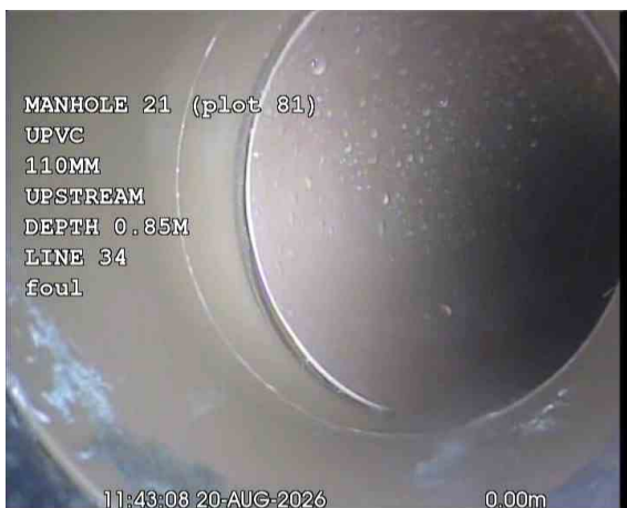
BASINX_6b07f886-8b8a-4975-912e-8edcb6200817_20260917_175748_246.jpg, 00:00:22, 0.00 m General remark, **PLOT 81**
