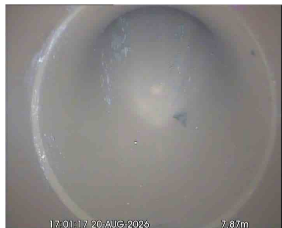
CAPPED OFFX_54005148-d235-4a76-8058-409ad506c306_20260918_101122_544.jpg, 00:00:34, 7.87 m Line deviates up, REST BEND
