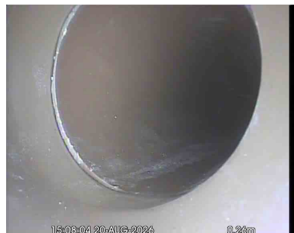
MH29X_dc951e00-981c-4e32-b78b-abbe7293dcb5_20260918_092732_216.jpg, 00:00:25, 0.26 m Line deviates right
