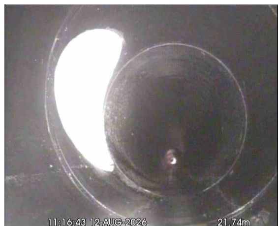
MH2 (S24)X_2b4372fb-7b8b-41ea-ad26-3972d5980a12_20260917_155917_684.jpg, 00:03:36, 21.74 m Junction at 9 o'clock, diameter: 150mm
