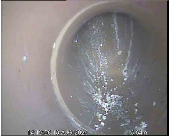
W_CX_b4296c61-451e-4780-b165-025cf86c2310_20260917_171113_525.jpg, 00:00:42, 3.54 m Line deviates up, REST BEND
