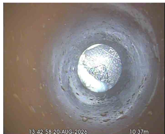
CAPPED OFFX_d02015fa-c904-4857-9e1b-08e97a9685ac_20260917_185409_523.jpg, 00:01:49, 10.37 m Survey abandoned, S/A - CAPPED OFF (WET ROOM)
