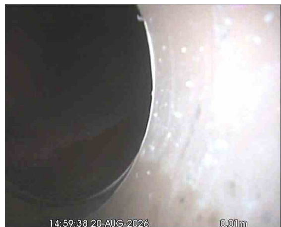
KIT. SINKX_0e666ae3-1ea5-4e19-80c1-67ada34d2ad5_20260918_091358_940.jpg, 00:00:23, 0.02 m Line deviates right
