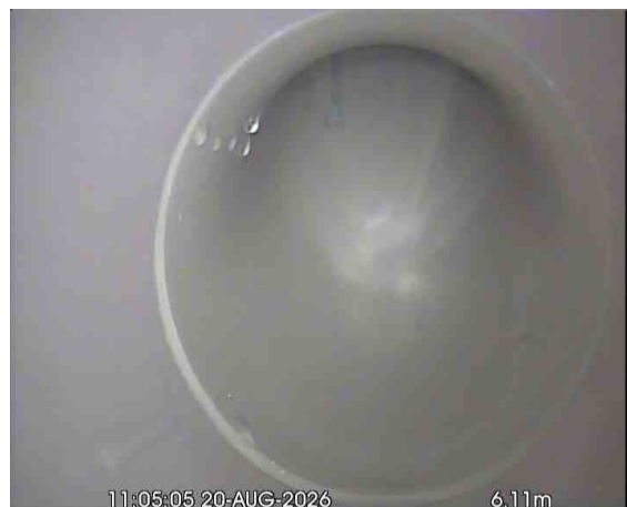
BASINX_3850f504-a288-4bef-9a1a-a2ea1de32231_20260917_173012_306.jpg, 00:01:12, 6.11 m Line deviates up, REST BEND
