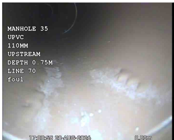
CAPPED OFFX_d53374e7-919c-4a41-9204-07a9a2f8a2ef_20260918_101042_084.jpg, 00:00:15, 0.00 m Start node, manhole, reference: MANHOLE 35 (MH35)
