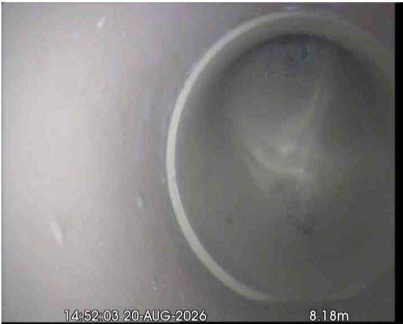
SVPX_8a9fe533-3cad-4b89-8ecf-f4aa226d6638_20260918_090909_460.jpg, 00:01:09, 8.18 m Line deviates up, REST BEND
