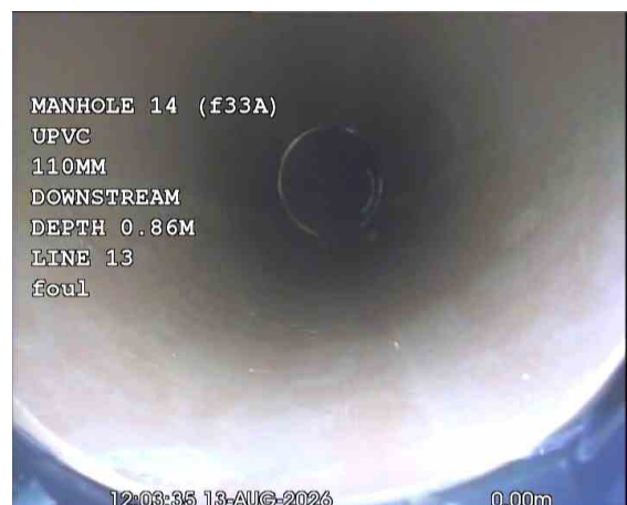
MH14 (F33AX_2c50aafe-6bcb-4f6c-a860-c40fdadf5679_20260917_165350_778.jpg, 00:00:34, 0.00 m Water level, 0% of the vertical dimension
