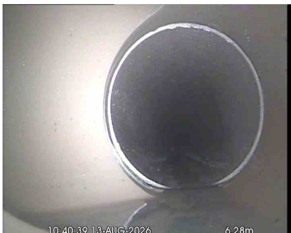
MH10 (F33)X_ab7df427-aa82-4b2d-aef8-1b8bd624a4aa_20260917_163020_967.jpg, 00:02:41, 6.28 m Junction at 9 o'clock, diameter: 110mm
