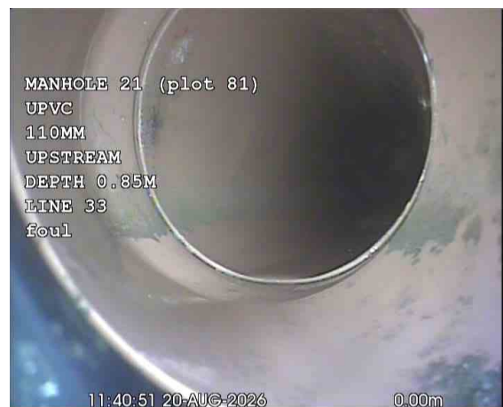
SVPX_57041f86-0a0d-4010-9a17-935acd425bad_20260917_175504_301.jpg, 00:00:40, 0.04 m Line deviates right
