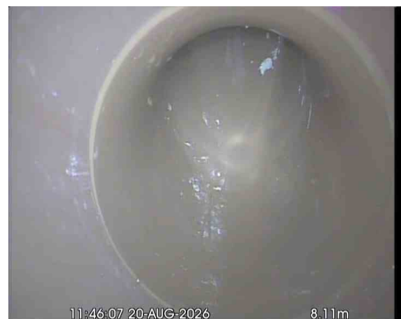
W_CX_ce8484da-cb17-481c-b19e-21035f4049d8_20260917_181545_839.jpg, 00:00:51, 8.11 m Line deviates up, REST BEND
