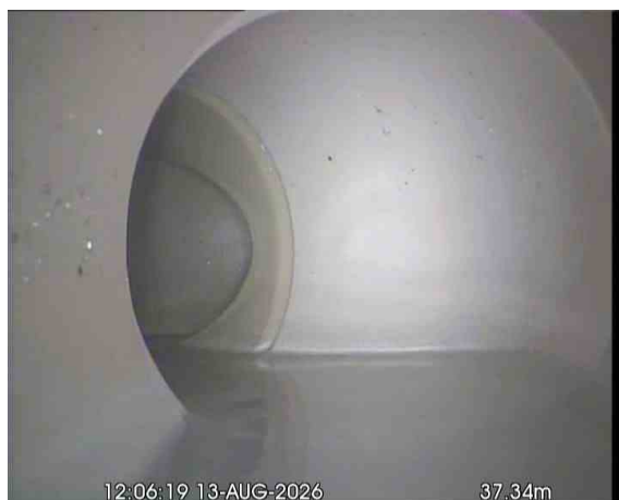
MH14 (F33AX_b46a8a86-547b-4291-951b-af5988893b71_20260917_165430_683.jpg, 00:03:18, 37.34 m Line deviates left
