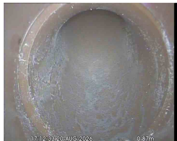
SVPX_953880e6-8502-4fde-9845-3e6edcb53494_20260918_101514_364.jpg, 00:00:30, 0.87 m Line deviates up, REST BEND
