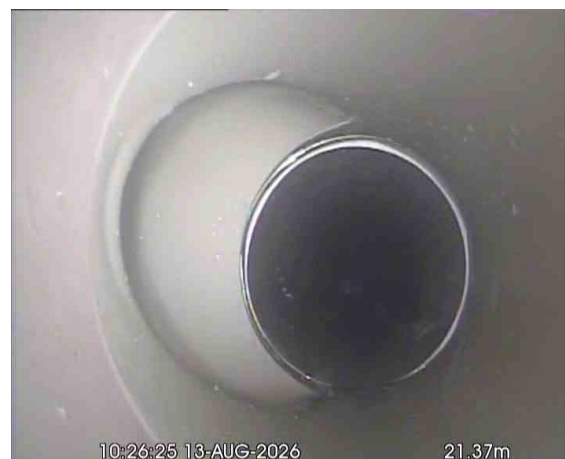
MH9 (F32)X_8025571e-a2ca-4ecc-98a6-1866d1e8da4c_20260917_162428_474.jpg, 00:03:19, 21.37 m Junction at 9 o'clock, diameter: 110mm
