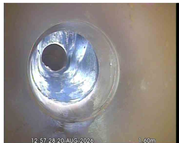
MH23X_c7c7f22a-c364-419f-9ab4-912108abca88_20260917_183936_624.jpg, 00:00:35, 1.60 m Line deviates left
