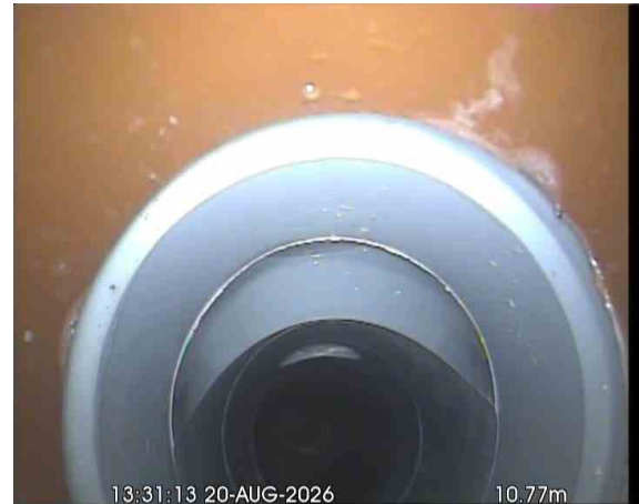
SVPX_06741d48-459e-47d2-b25c-0dd297d9ba21_20260917_184703_127.jpg, 00:01:27, 10.77 m Finish node, major connection without manhole, reference: SOIL VENT PIPE (SVP) & DOWNSTAIRS W/C
