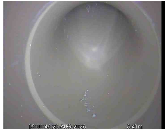
KIT. SINKX_62ebc3ac-0d35-4160-b030-966308e9e49c_20260918_091441_704.jpg, 00:00:36, 3.41 m Line deviates up, REST BEND
