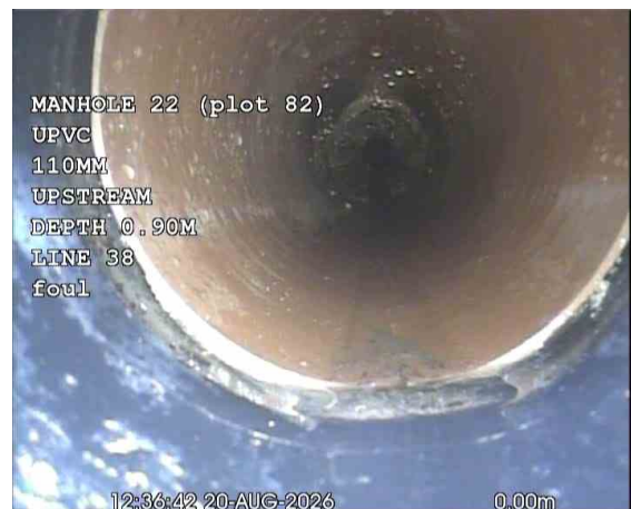
SVPX_42910abf-b3e8-4d00-8c7a-8bd7cd52181b_20260917_182957_373.jpg, 00:00:15, 0.00 m Water level, 0% of the vertical dimension
