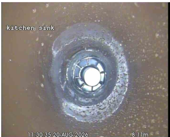
KIT. SINKX_a991a2f0-69f1-4353-b84d-bd3e5162529b_20260917_174934_935.jpg, 00:01:20, 8.11 m Finish node, major connection without manhole, reference: KITCHEN SINK
