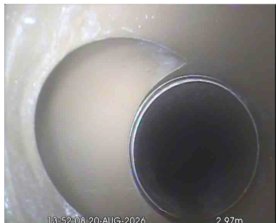
MH26X_fa2cfba1-3b82-4303-a741-1397692fa505_20260917_185813_273.jpg, 00:01:15, 2.97 m Junction at 9 o'clock, diameter: 110mm, SECTION 52 (S52)
