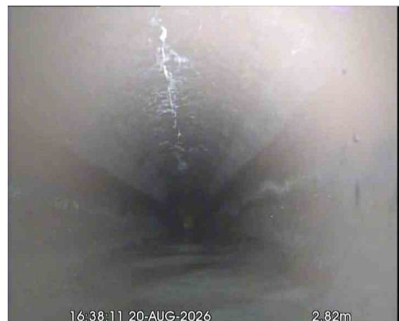
MH32X_f05a7949-5f1b-43ac-a906-2a5c79c411e9_20260918_095215_718.jpg, 00:00:38, 2.82 m Water level, 10% of the vertical dimension
