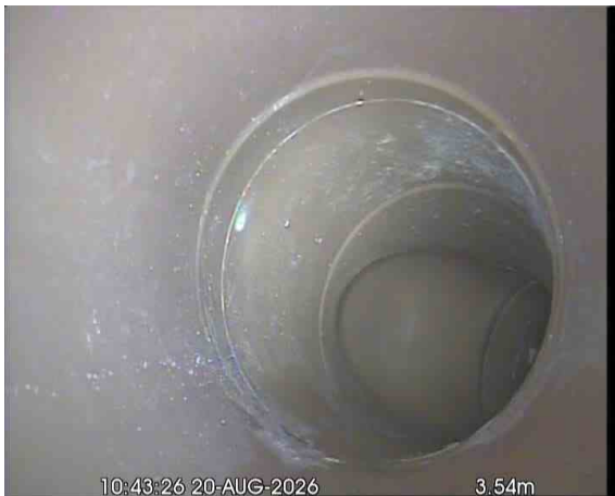
MH18X_268b6589-d669-4bfe-9c9b-40feec28391f_20260917_172703_203.jpg, 00:00:53, 3.54 m Line deviates right
