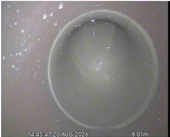
CAPPED OFFX_7f4e235e-2145-42ce-9168-67b113218515_20260918_090712_645.jpg, 00:01:05, 8.01 m Line deviates up, REST BEND
