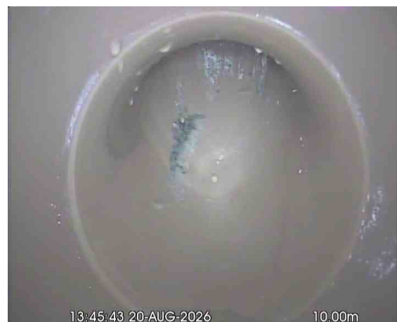
SVPX_1f7c8f2b-79d4-4b84-8986-45f786409ac9_20260917_185533_394.jpg, 00:01:07, 10.00 m Line deviates up, REST BEND
