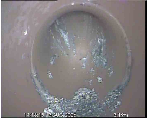
BASINX_f79740ec-7974-48e7-9a37-fc3e2b8576cc_20260917_170920_384.jpg, 00:00:58, 3.19 m Line deviates up, REST BEND
