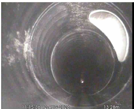
MH2 (S24)X_6d0cafe9-aaba-4e45-9438-a7dde209d2f5_20260917_155841_148.jpg, 00:02:29, 13.28 m Junction at 2 o'clock, diameter: 150mm
