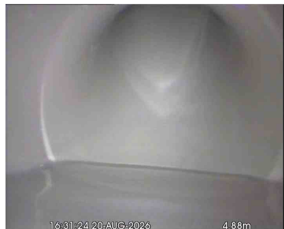
SVPX_649224af-f3da-49ce-90a6-0e9e9bcac291_20260918_094533_662.jpg, 00:01:27, 4.88 m Line deviates up, REST BEND
