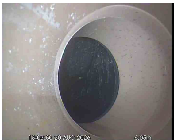
MH24X_05513c93-b7d8-4673-ac1b-77e9709ec39b_20260917_184206_762.jpg, 00:01:22, 6.05 m Line deviates left
