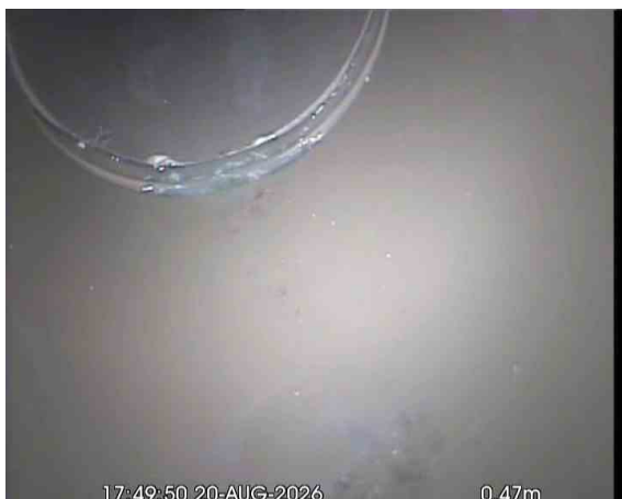
MH39X_f79daff0-11d6-4245-905a-5bf3eafa14c5_20260918_103525_006.jpg, 00:00:38, 0.47 m Line deviates up
