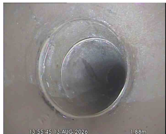
SVPX_522d8c10-0f75-4268-8945-1182ee759427_20260917_165750_365.jpg, 00:00:41, 1.88 m Line deviates right
