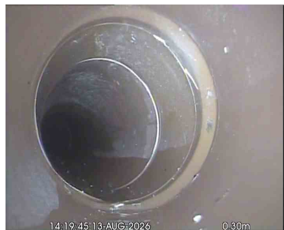
W_CX_a57f05f7-9d6c-4b65-8ab5-76ee476a6623_20260917_171049_396.jpg, 00:00:29, 0.30 m Line deviates left
