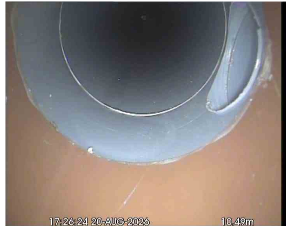
SVPX_f5f94117-bd53-44f6-ba76-d325dfd2f447_20260918_102439_810.jpg, 00:01:17, 10.49 m Finish node, major connection without manhole, reference: SOIL VENT PIPE (SVP) & KITCHEN SINK
