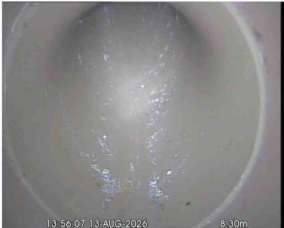
SVPX_9d28b386-32ca-434f-a99a-b130670ade5b_20260917_165803_576.jpg, 00:01:04, 8.30 m Line deviates up, REST BEND
