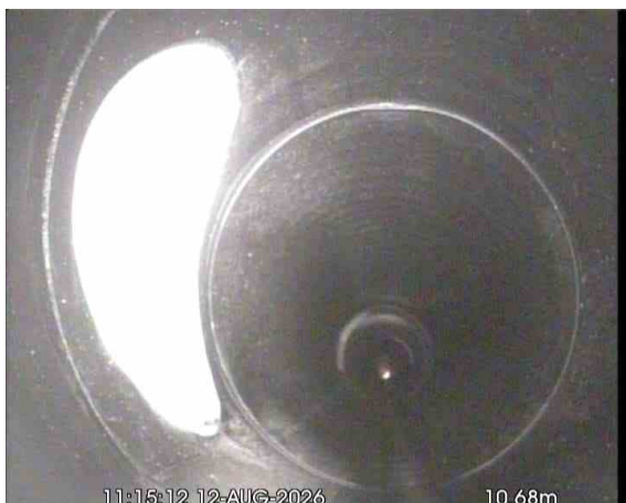
MH2 (S24)X_9bc9b007-b930-48ab-9bd4-88c17d308de9_20260917_155756_854.jpg, 00:02:05, 10.68 m Junction at 9 o'clock, diameter: 150mm
