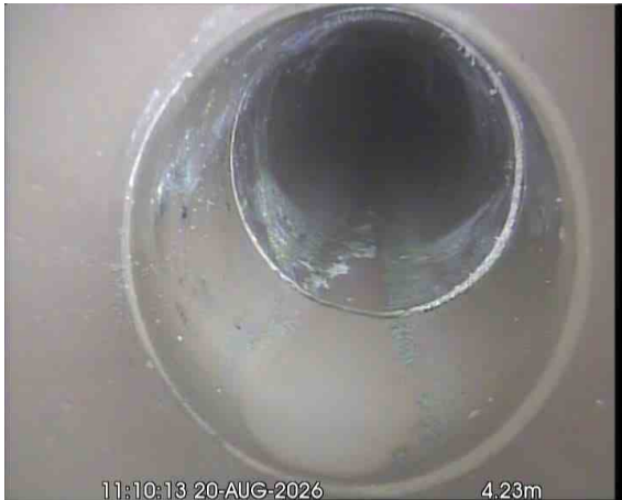
MH19X_d9462d28-2e68-4964-8066-9cb3c1f9aded_20260917_173541_582.jpg, 00:01:14, 4.23 m Line deviates up
