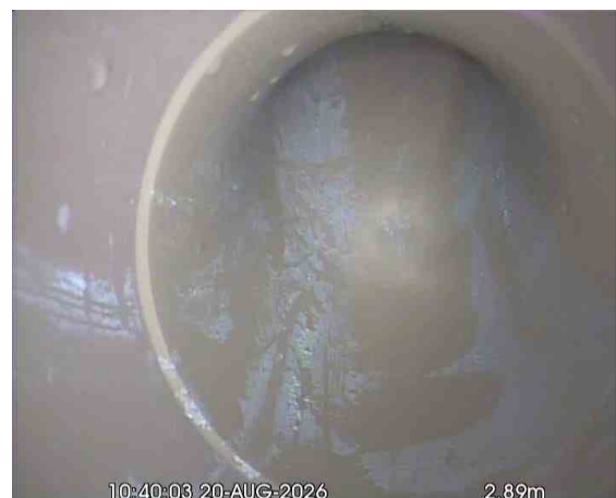
SVPX_6b41b416-6a39-4cfe-a2c1-4a535335776f_20260917_172508_036.jpg, 00:01:04, 2.89 m Line deviates up, REST BEND
