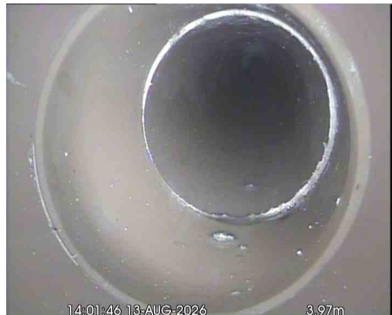
MH15X_87962072-6ce7-428c-a931-a891d0940a54_20260917_170250_140.jpg, 00:00:59, 3.97 m Line deviates up
