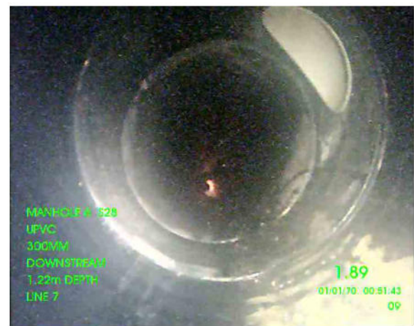
MH6 (S28)X_f57b6097-6d31-4ada-8367-ff2e3ea0c0ce_20260917_161451.png, 1.89 m Junction at 2 o'clock, diameter: 150mm
