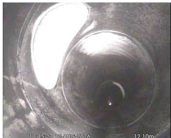
MH2 (S24)X_95af4d62-58af-4330-bcfa-b7b9eaa6bf5f_20260917_155813_356.jpg, 00:02:20, 12.10 m Junction at 10 o'clock, diameter: 150mm
