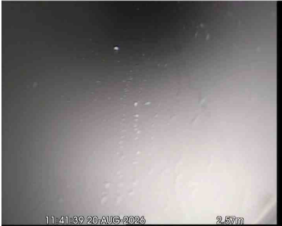
SVPX_098eba58-6aa0-40bd-a60f-874d1c9b9a5d_20260917_175641_405.jpg, 00:01:27, 2.57 m Finish node, major connection without manhole, reference: SOIL VENT PIPE (SVP)
