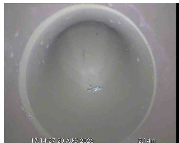
CAPPED OFFX_9192abd0-fe56-4978-b900-76fe471a808c_20260918_101850_913.jpg, 00:00:30, 2.14 m Line deviates up, REST BEND
