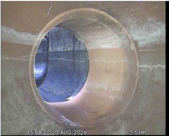
MH29X_b1b87763-5835-4bce-891d-8157de740b19_20260918_092750_310.jpg, 00:00:42, 5.51 m Line deviates left
