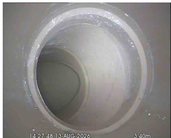
MH17X_1142224a-fbc7-4b73-ae62-4d6160c99412_20260917_171541_910.jpg, 00:01:36, 3.40 m Line deviates left
