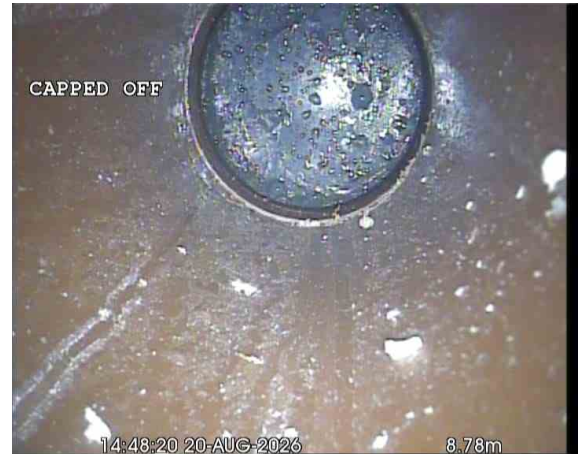
CAPPED OFFX_1bbbbbf9-df29-4d90-86ab-ff12e9751df9_20260918_090734_766.jpg, 00:01:21, 8.78 m Survey abandoned, S/A - CAPPED OFF (WET ROOM)
