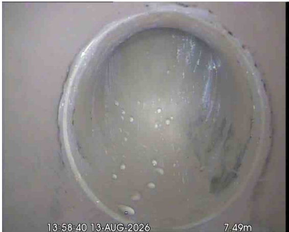
UTIL. SINKX_5626fec3-1c3c-4485-a61d-6a0c0dc85c02_20260917_170008_894.jpg, 00:00:57, 7.49 m Line deviates up, REST BEND
