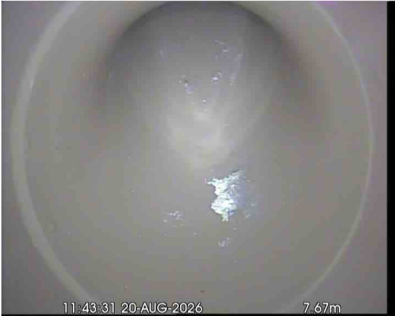
BASINX_f196327a-540f-41ef-960d-920cd33a2aef_20260917_175813_068.jpg, 00:00:46, 7.67 m Line deviates up, REST BEND
