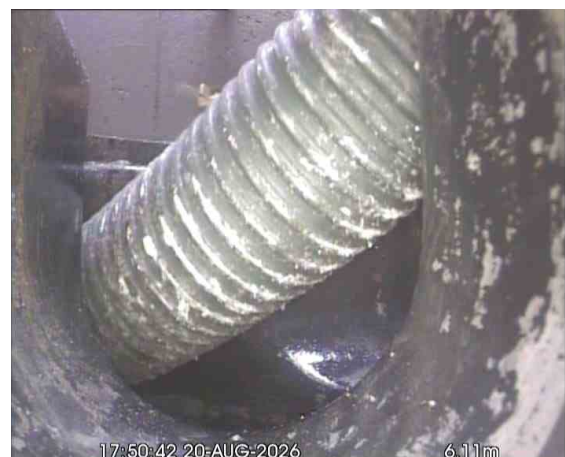
MH39X_e549956b-95b0-40d2-bfe8-acef5b96bd59_20260918_103628_466.jpg, 00:01:24, 6.11 m Finish node, manhole, reference: MANHOLE 11 (MH11) - IN THE ROAD, (F34)
