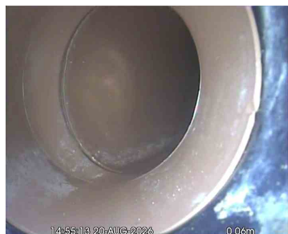
MH28X_dceb120e-1642-4f0e-b11c-9d226030ae20_20260918_091155_748.jpg, 00:00:27, 0.06 m Line deviates right
