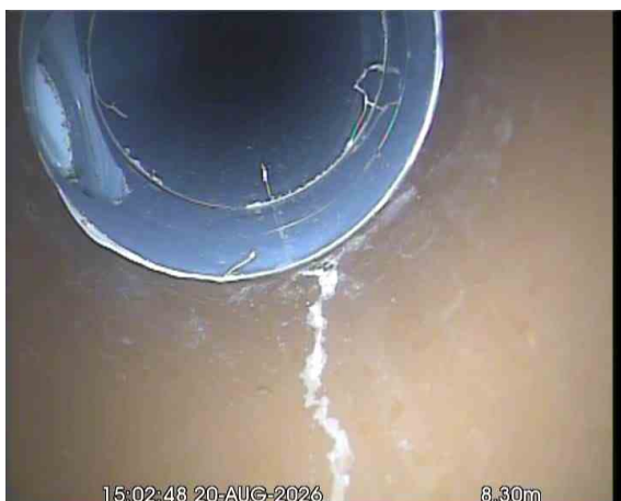
SVPX_e8fae199-0d18-40df-852d-9152b1a3257f_20260918_092144_539.jpg, 00:01:00, 8.30 m Finish node, major connection without manhole, reference: SOIL VENT PIPE (SVP) & UTILITY SINK
