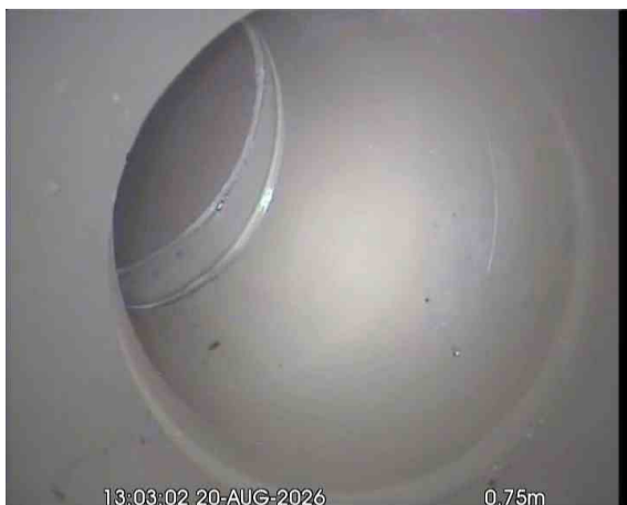
MH24X_e51a6242-5226-4a44-904b-1452dcda3dea_20260917_184139_287.jpg, 00:00:39, 0.75 m Line deviates left
