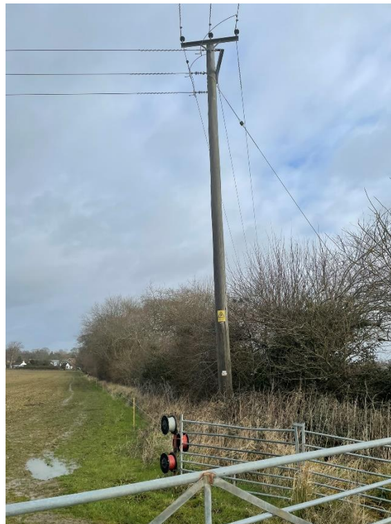
Photo 4: Gateway and overhead cable sand pole showing the junction cable heading northeast
