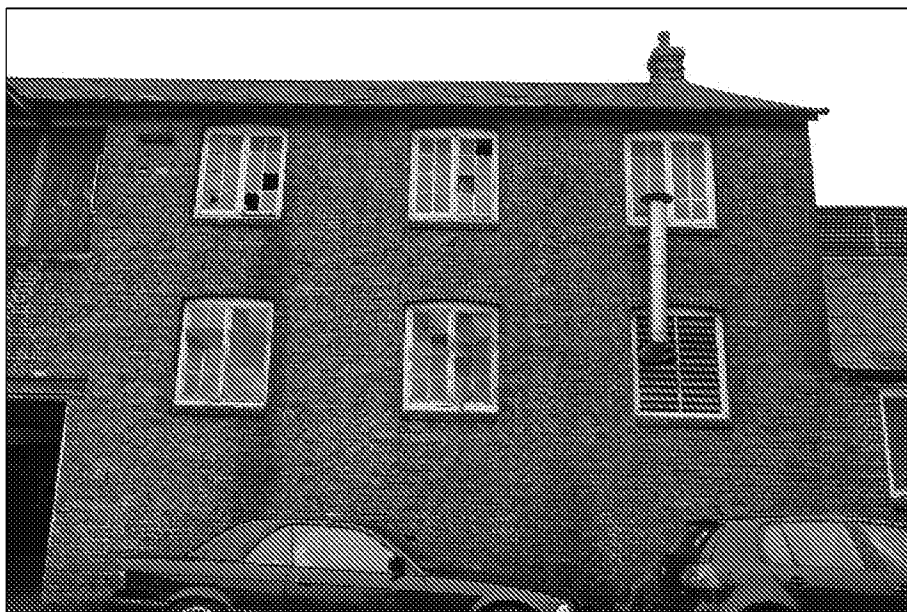
Figure 15: View looking west towards northern extent of two-storey range where casement 16-light segmental arch timber-framed windows have been damaged, or replaced with modern louvers and plant.
