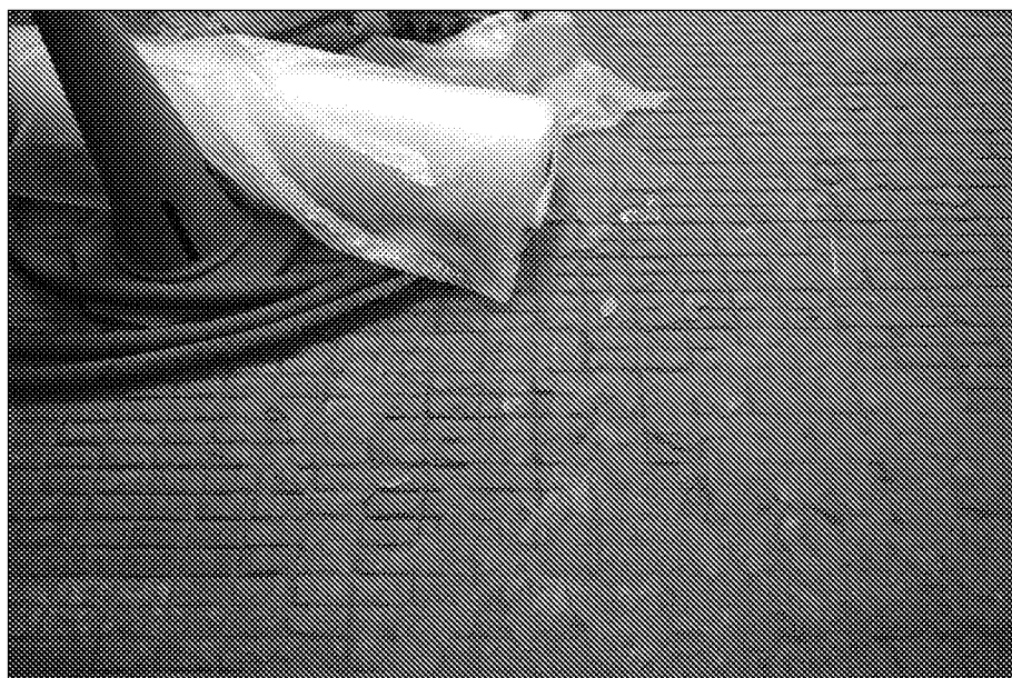
Figure 21: Engineering brick floor patched up with modern concrete.
