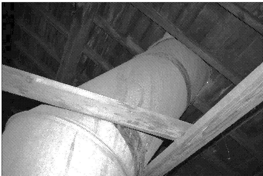
Figure 29: Modern metal flue which has been inserted from ground floor plant room below and out through planked underside of roof.
