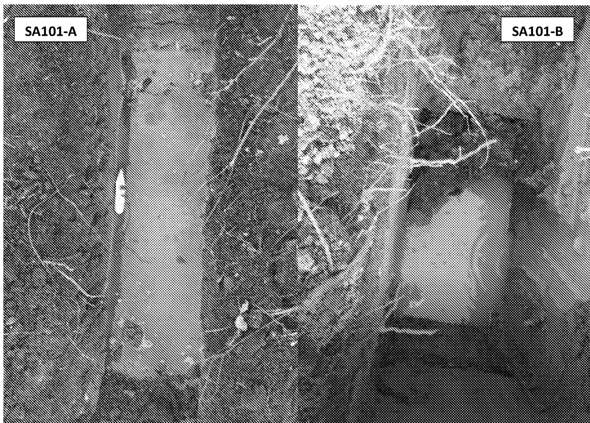
PLATE 2: Trial pits SA101-A and SA101-B showing groundwater ingress after excavation.
