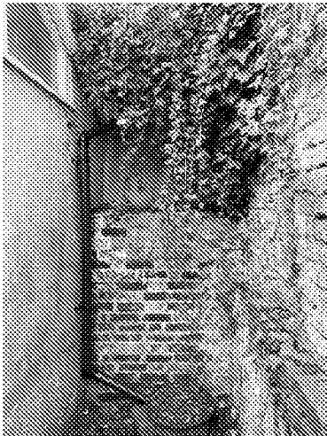
Photo No. 11 - Return wall to the West side of the rear retaining boundary wall. Drainage to the roof over the building
