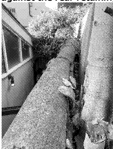
Photo No. 15 – Cracked concrete capping and movement to the top of the rear retaining boundary wall at the location of the tree within the back garden of Newburgh House
