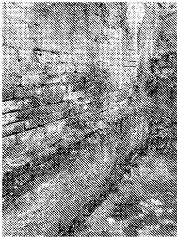
Photo No. 3 – Rear retaining boundary wall. Note vegetation growing against the wall
