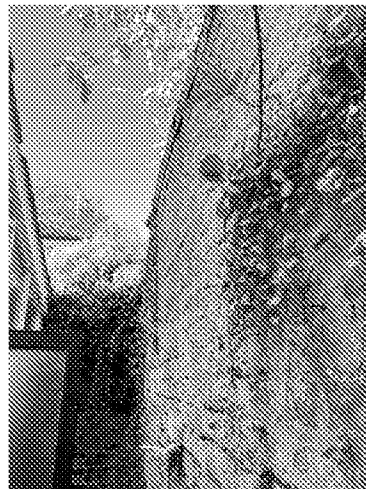
Photo No. 4 – Bulging and leaning at high level to the rear retaining boundary wall
