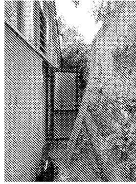
Photo No. 2 – Rear retaining boundary wall. Note vegetation growing against the wall
