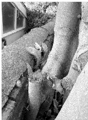
Photo No. 14 – Tree within the back garden of Newburgh House growing directly against the rear retaining boundary wall
