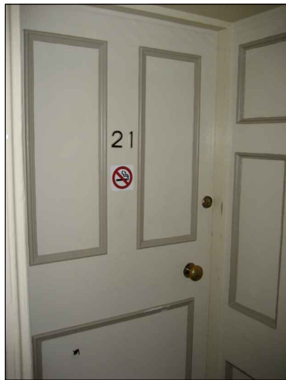
Existing Bedroom 21 Door with applied beading.
