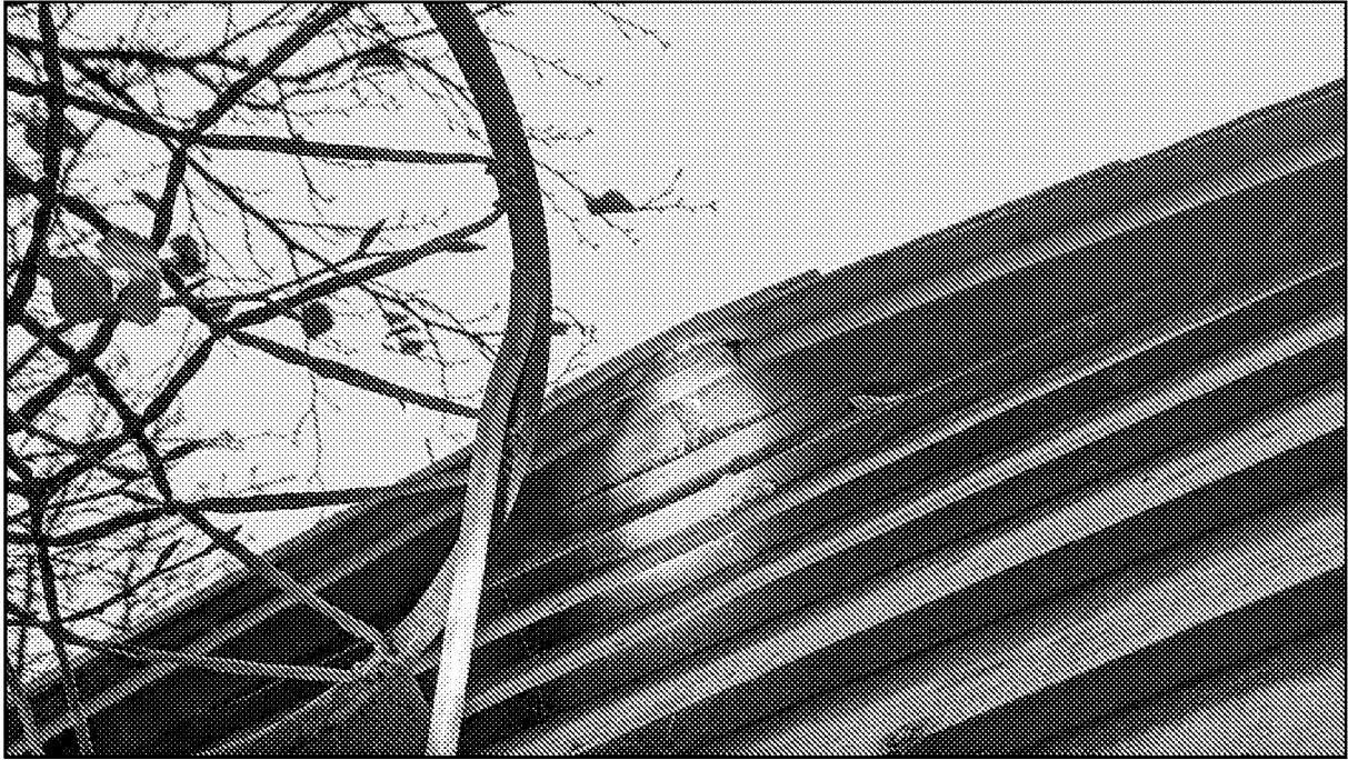
Photo 5 – Closeup showing gaps along the gable end.
