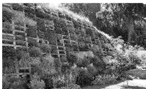
Image of planted crib retaining wall system
