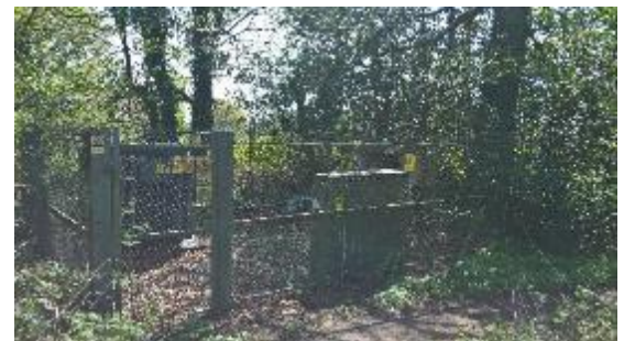
Plate 9.8: Electricity substation in south-eastern corner of site
