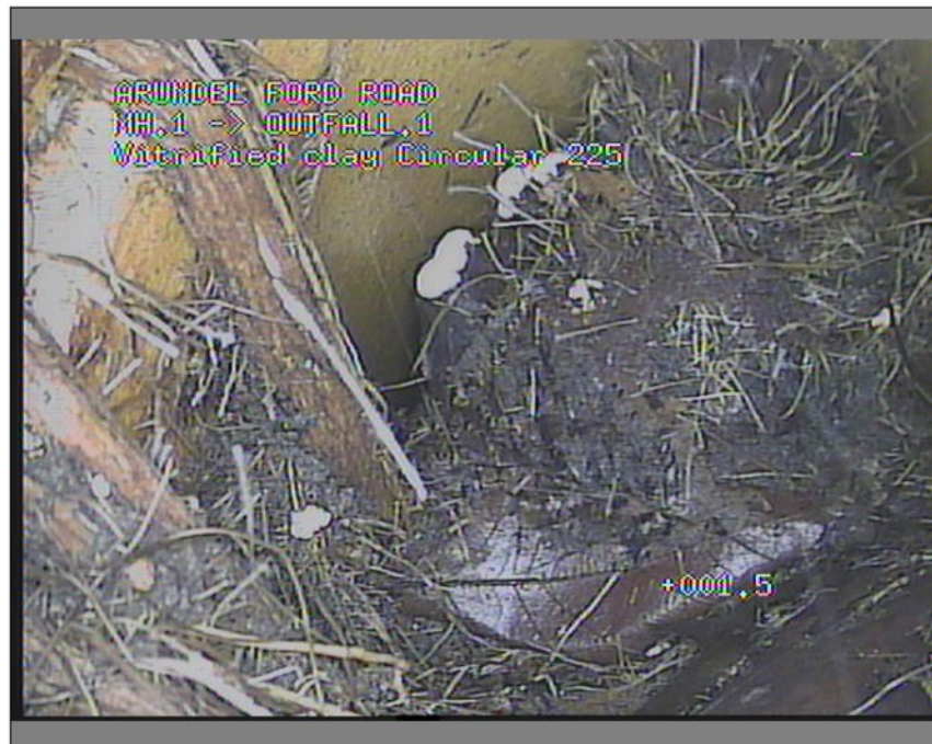
Photo: 6_6_54_A.JPG 1.5m, Roots, tap at joint
