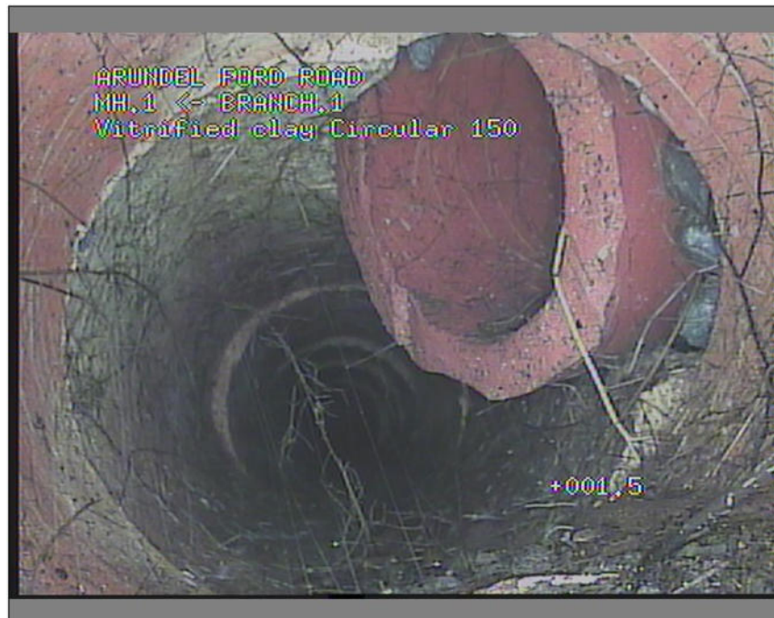
Photo: 4_4_17_A.JPG 1.5m, Connection intruding, at 2 o'clock, diameter 100mm, intrusion 40%
