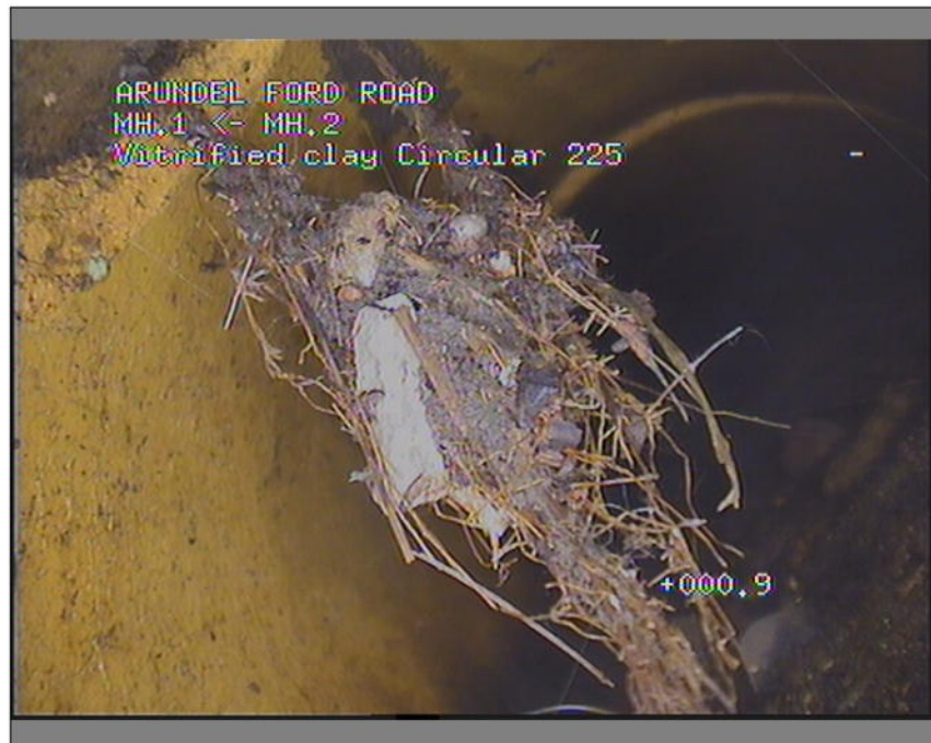
Photo: 1_1_6_A.JPG 0.9m, Roots, mass, 10% cross-sectional area loss
