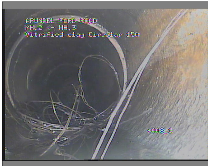
Photo: 8_8_70_A.JPG 8.1m, Roots, mass at joint, 10% cross-sectional area loss
