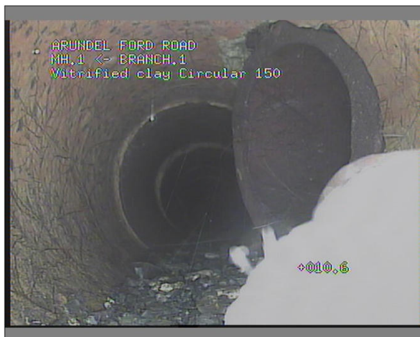
Photo: 4_4_21_A.JPG 10.6m, Connection intruding, at 3 o'clock, diameter 150mm, intrusion 30%
