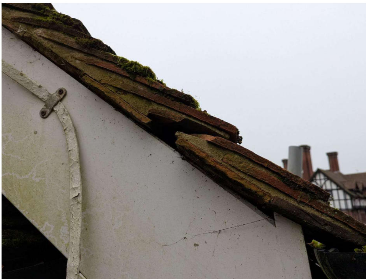
Figure 3.3.1- cracked tile capping and adhered bat dropping immediately below.
