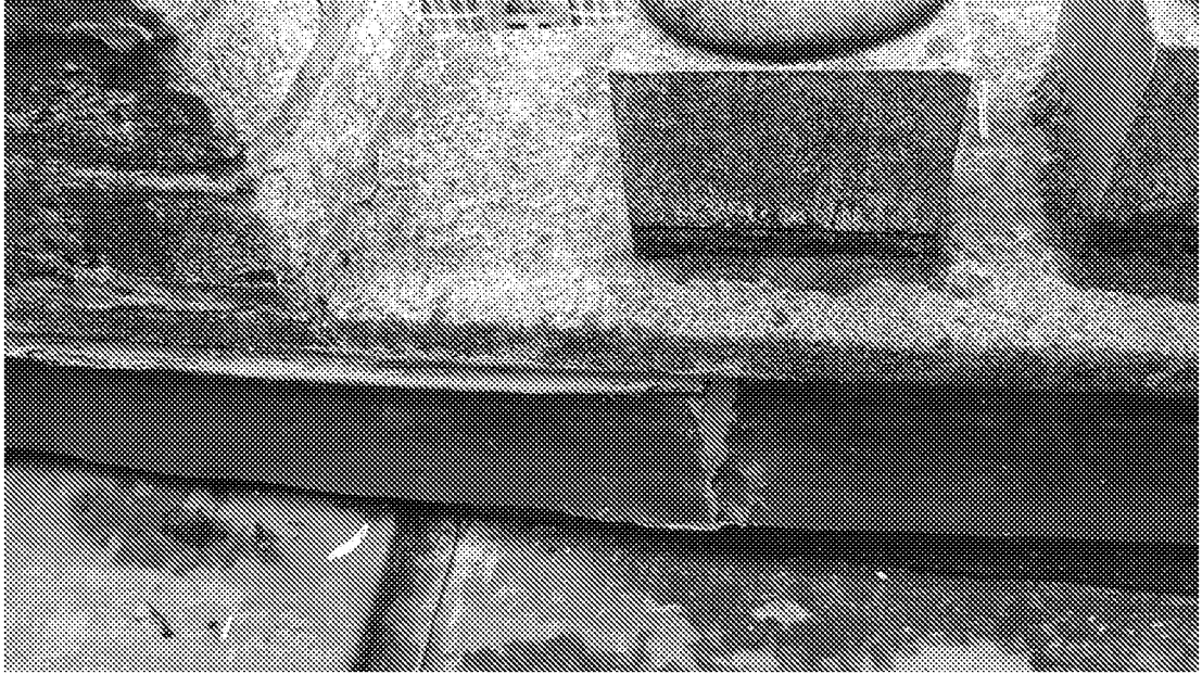
Crack in concrete wall of the building
