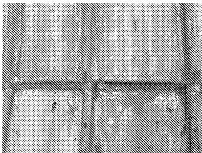
Typical image of one of the many holes and creases in the lead
