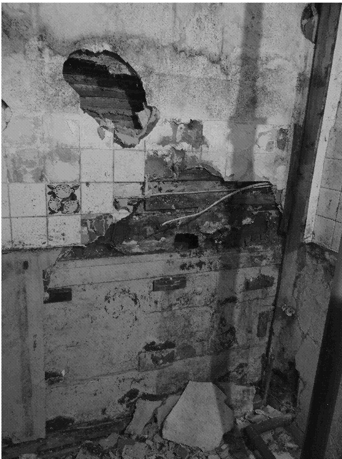
Party wall damage
