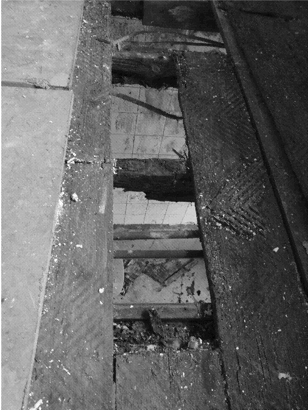
Floor board damage
