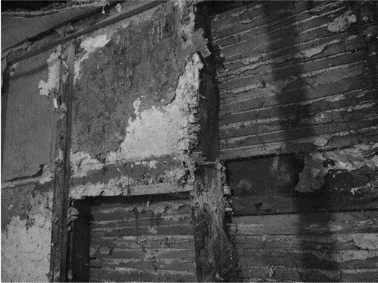
More party wall damage evidence
