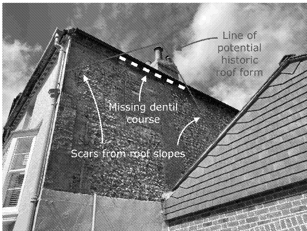
Scarring, with what appears to be an associated length of missing dentil course, suggests a potential historic roof and a building which would have continued the historic grain along the current line.
