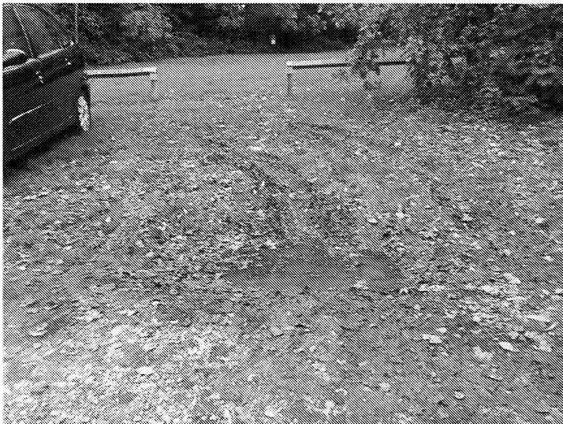
Photo 8: Condition of the off road parking area 17th October 2014
