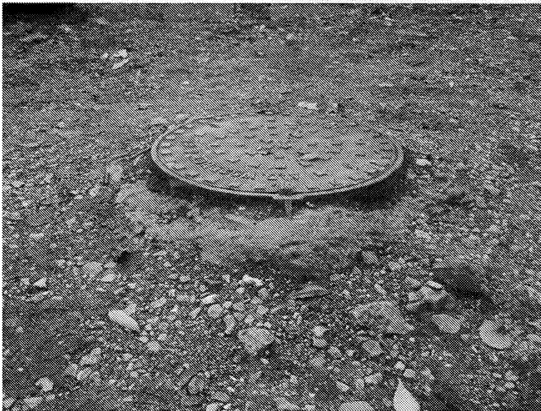
Photo 7: Exposed manhole cover in the off road parking area 19th October 2014
