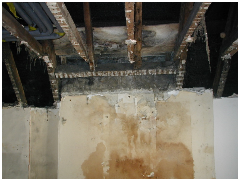
Picture – Roof structure showing signs of water ingress and deterioration.
