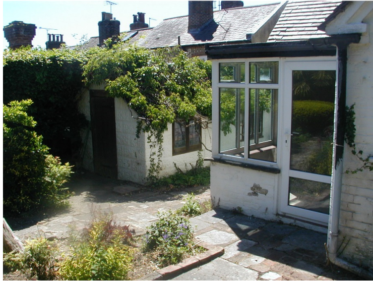
Picture – Garage with roof overgrown with Ivy.
