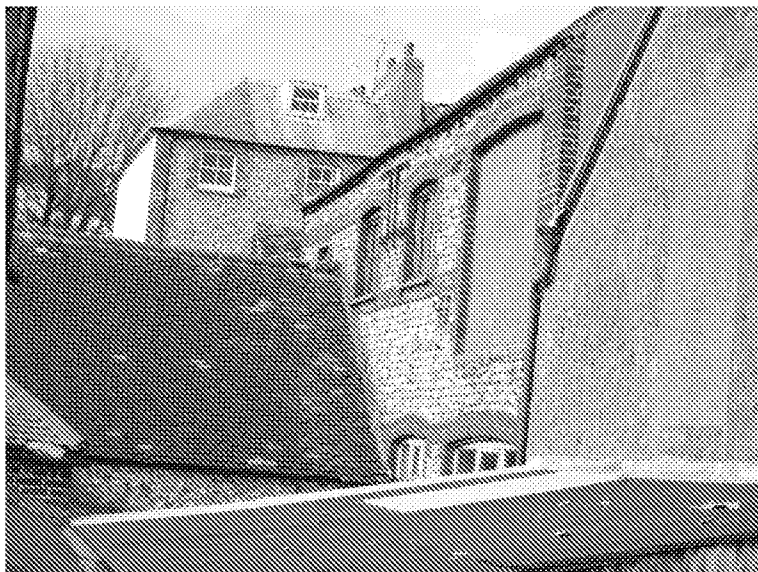
Figure 1 - West flank wall of Building 1 and rendered gable of Building 2. Note wall and roof construction, together with bulging wall line at roof level.
