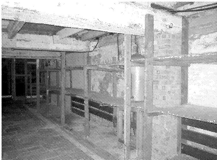
Figure 8 - Looking west on the ground floor of Building 3, illustrating propped first floor beam and water entry. Retaining wall is to right of photograph.
