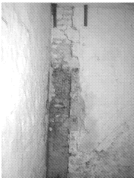
Figure 4 - Cracking on first floor level in south east corner, flank wall to left of picture
