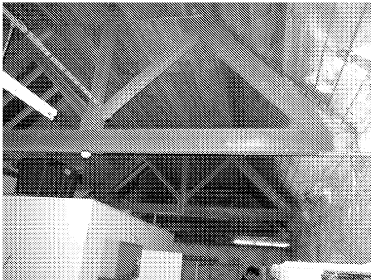
Figure 7 - Looking east in Building 3, indicating roof structure and water entry
