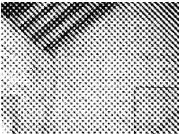
Figure 2 - North West Corner Cracking and Wallplate Movement
