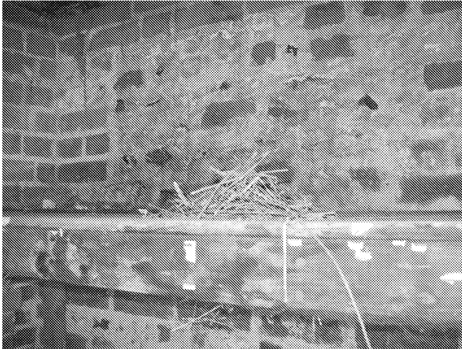
Photograph 4.1: Evidence of breeding birds in the two storey brick and flint building to the west of the site.
