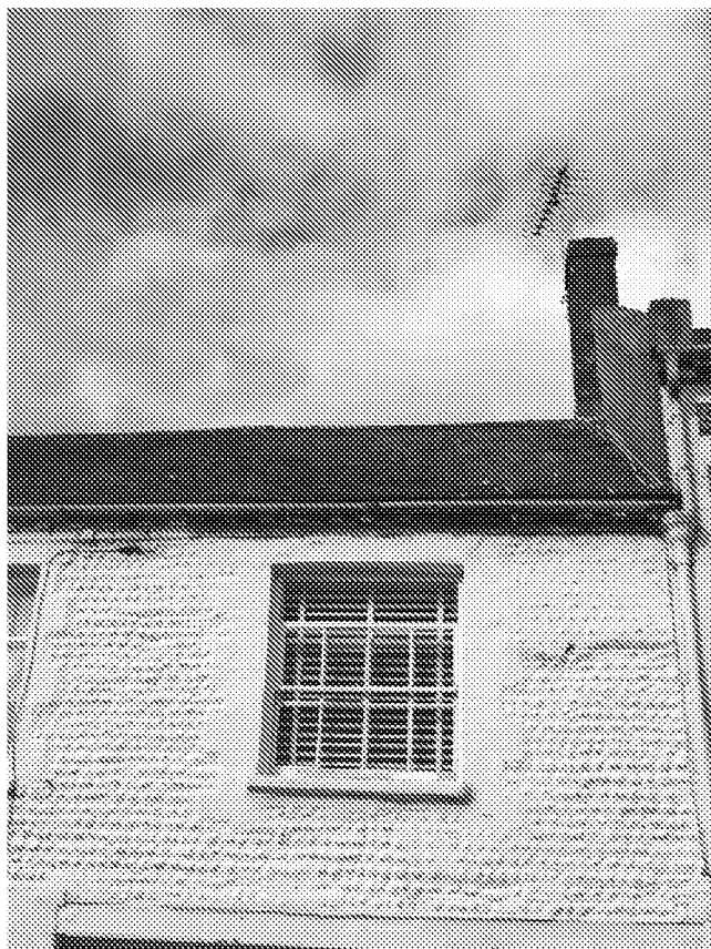
Further close up of failing flint mortar
